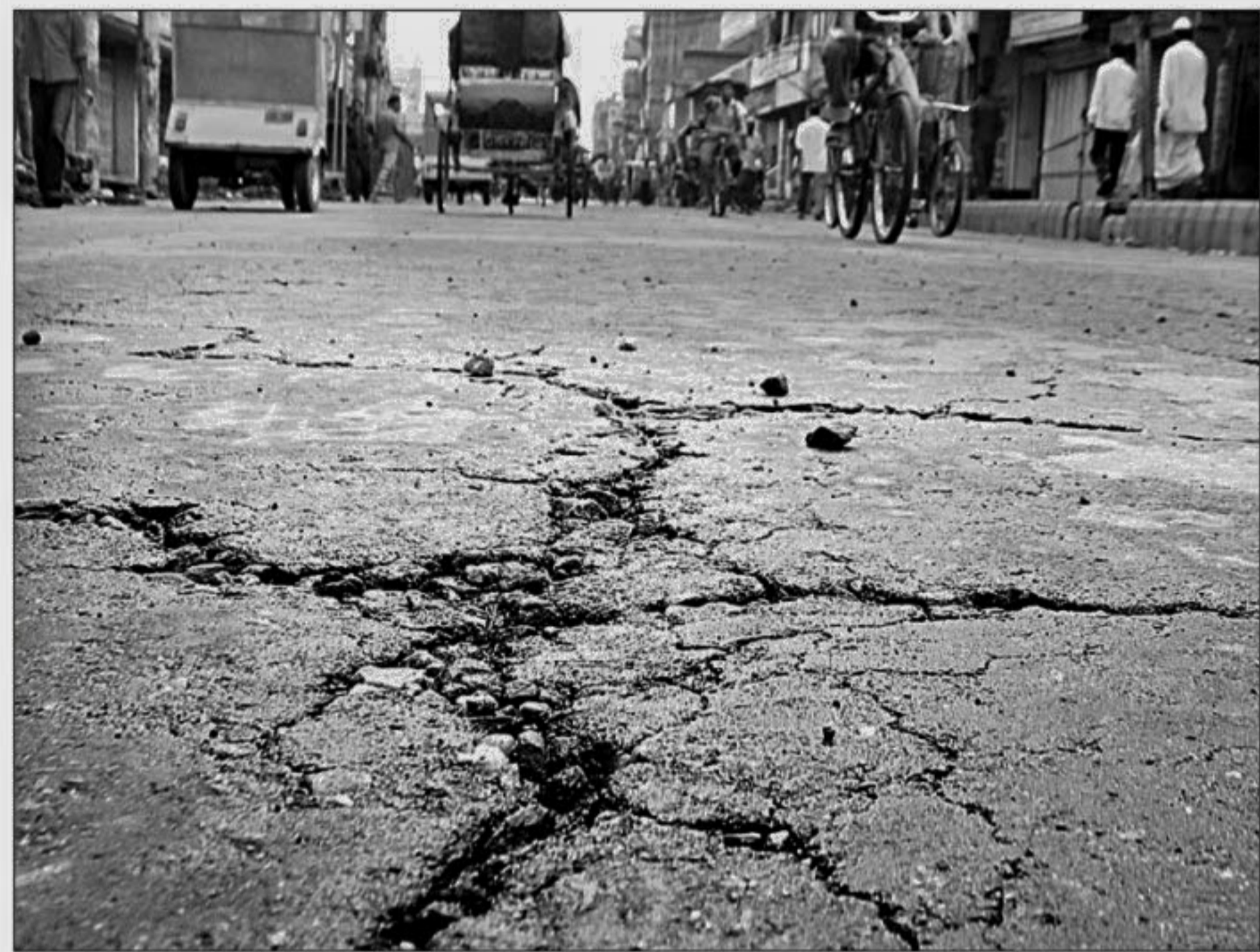
Large cracks develop on Birshreshtha Capt Mohiuddin Jahnagir road in Barisal town only after five months of its renovation early this year. The photo was taken recently.
