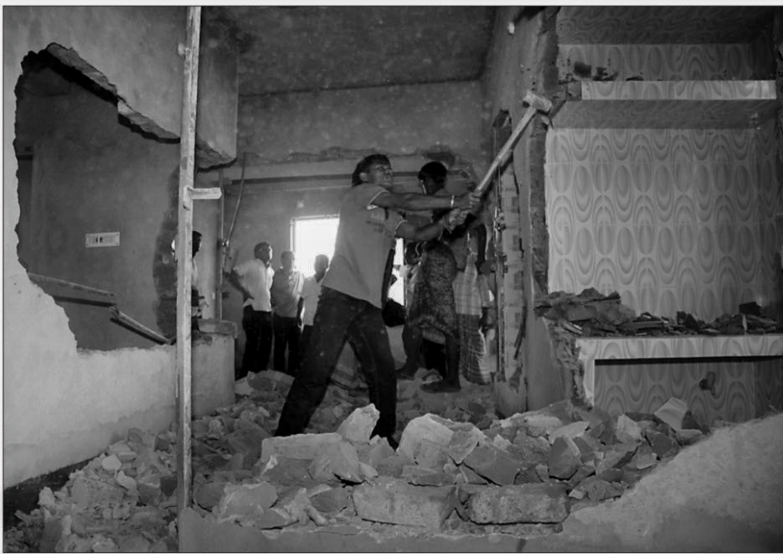
Rajdhani Unnayan Kartripakkha (Rajuk) starts knocking down a seven-storey illegal building in the city's east Begunbari yesterday. (Story on Page 1)
