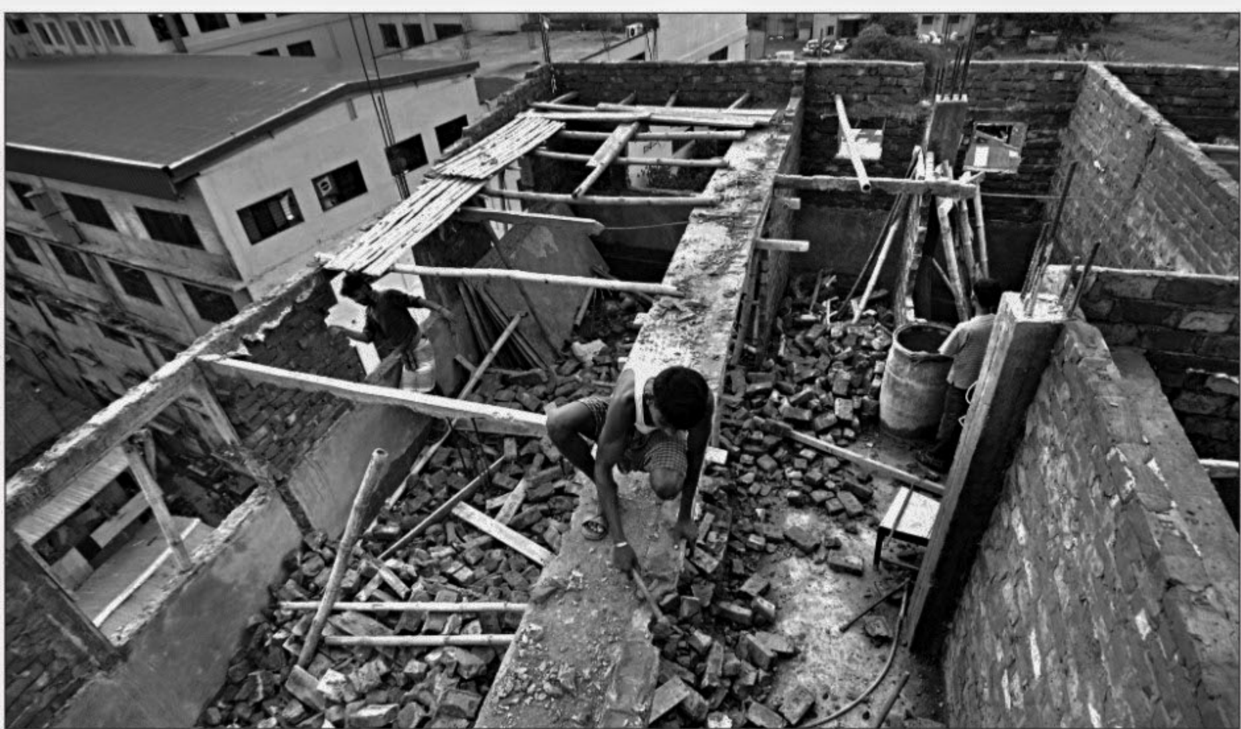
Workers start demolishing a tilted house at Begunbari in the city yesterday after Rajdhani Unnayan Kartipakkha served a notice to its owner for demolition of the house. The seven-storey building tilted on Friday, creating panic among its residents and their neighbours.
