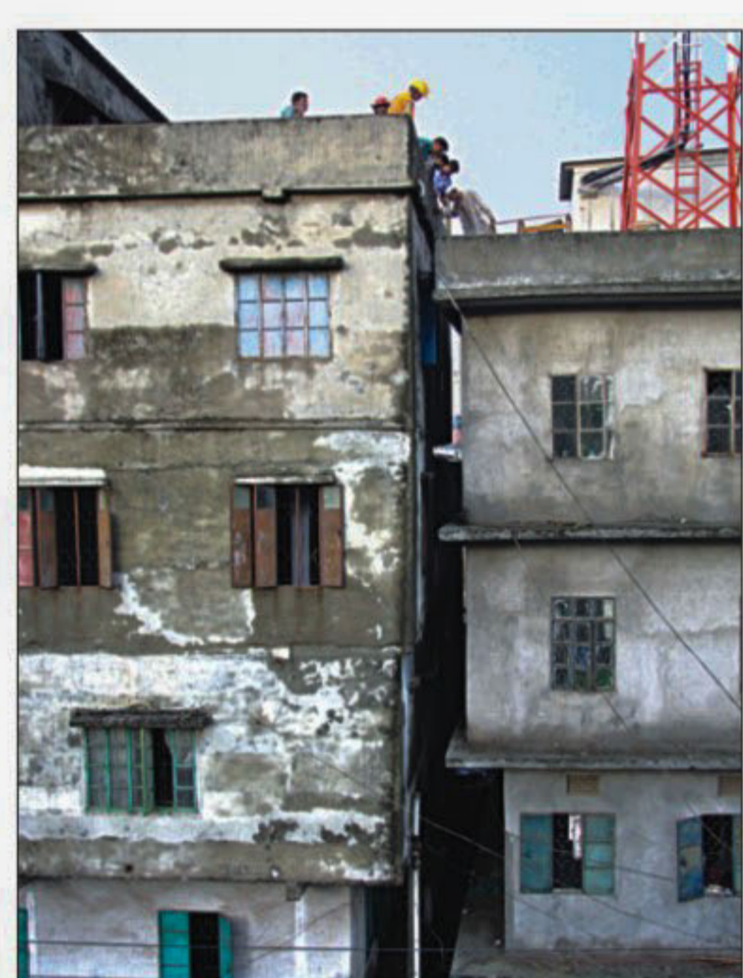
A four-storey building at the city's Nakhapara tilts to one side yesterday afternoon. The sudden leaning of the structure spread a wave of panic through the area as the memory of Tuesday night's building collapse at Begunbari is still fresh among the city dwellers.
