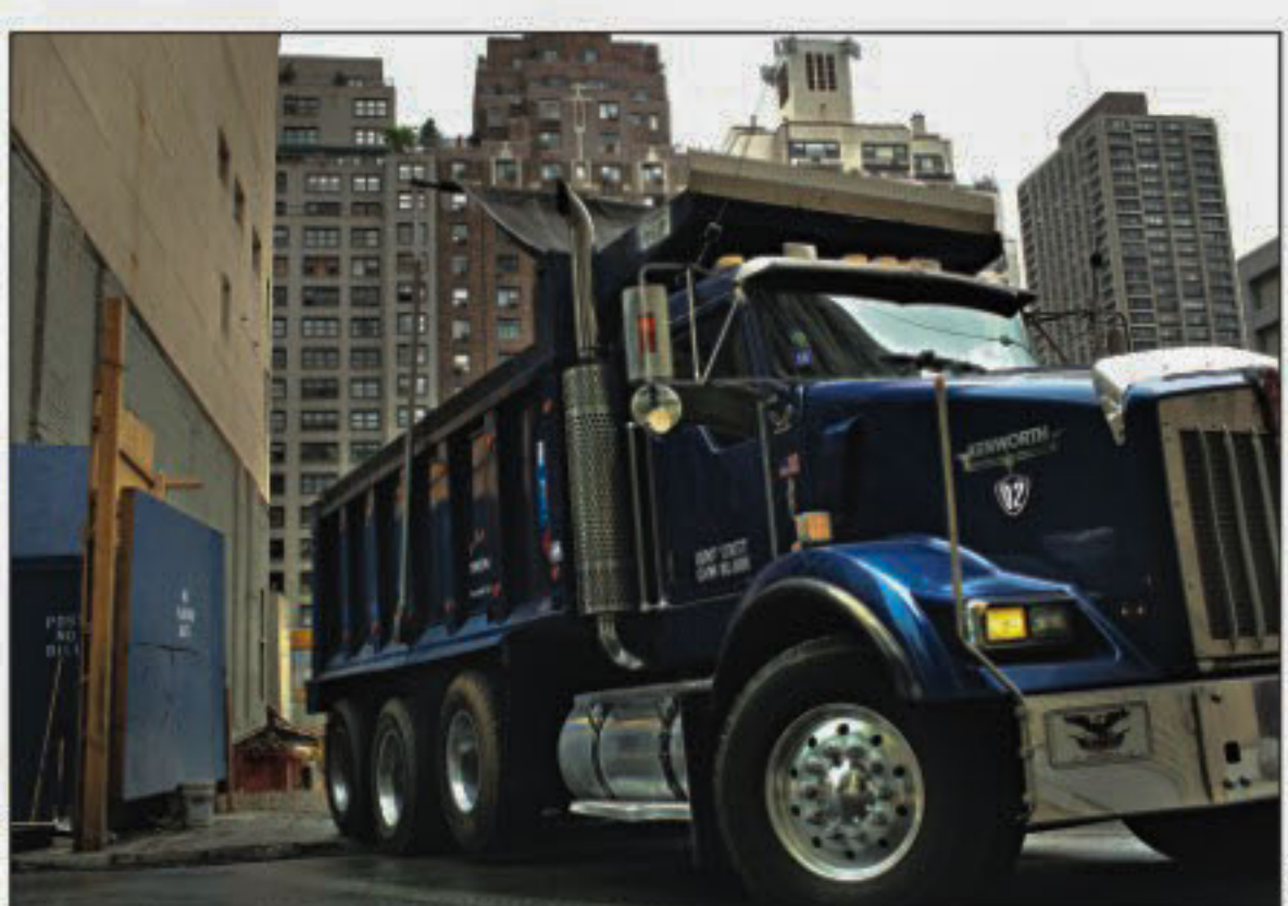
A truck pulls out of a construction site, which had been halted due to the economic recession and the slowdown in the real estate market on 57th street on Thursday in New York City. The site will eventually house a Whole Foods among other businesses. As the economy gradually improves, hundreds of once dormant construction projects in New York City are beginning to start up again.
