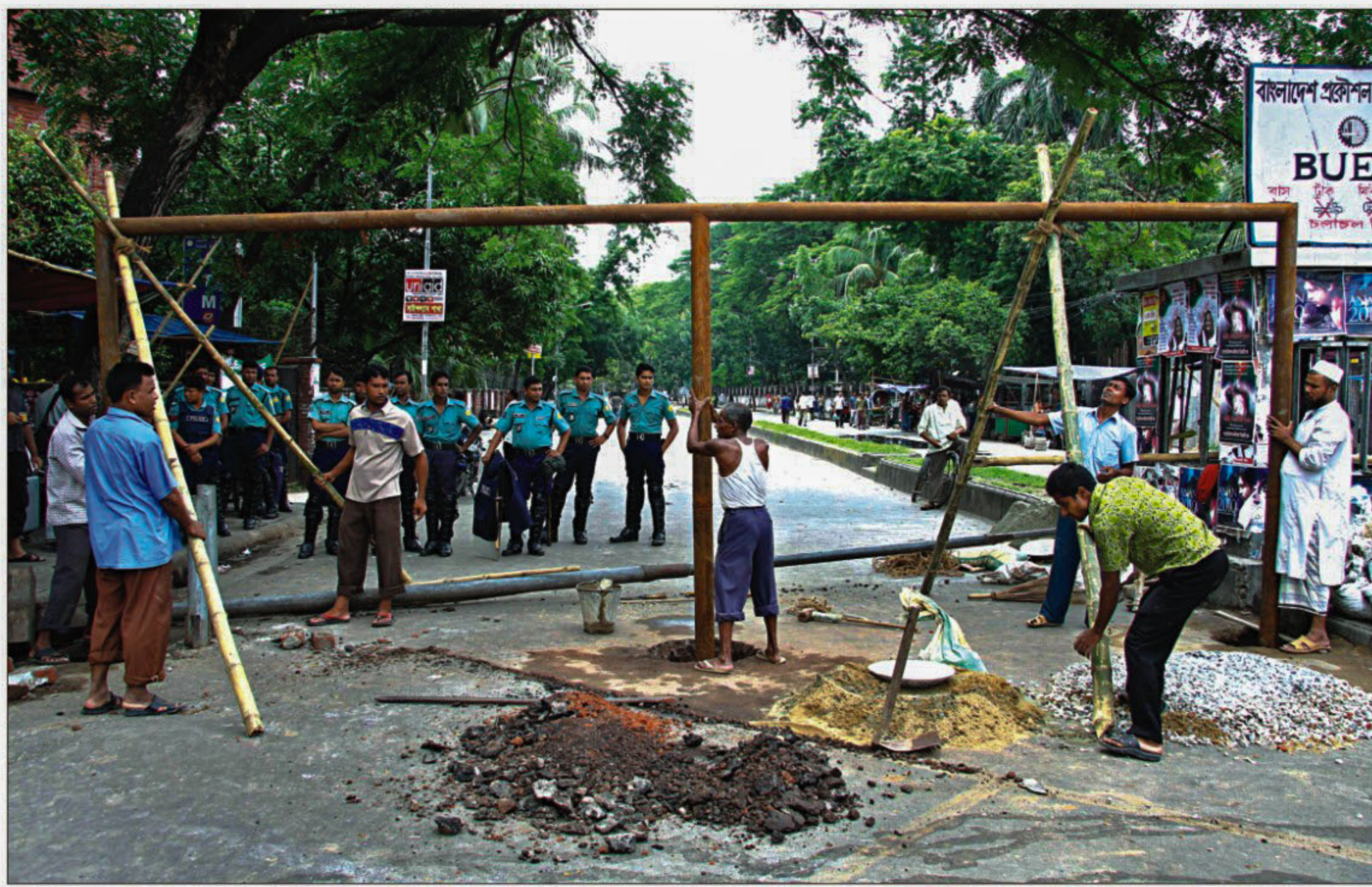
Workers install vehicle height restrictor at Palashi in the capital yesterday. Buet authorities decided to install the restrictor after a recklessly driven bus fatally ran over a student the day before. PHOTO: STAR
