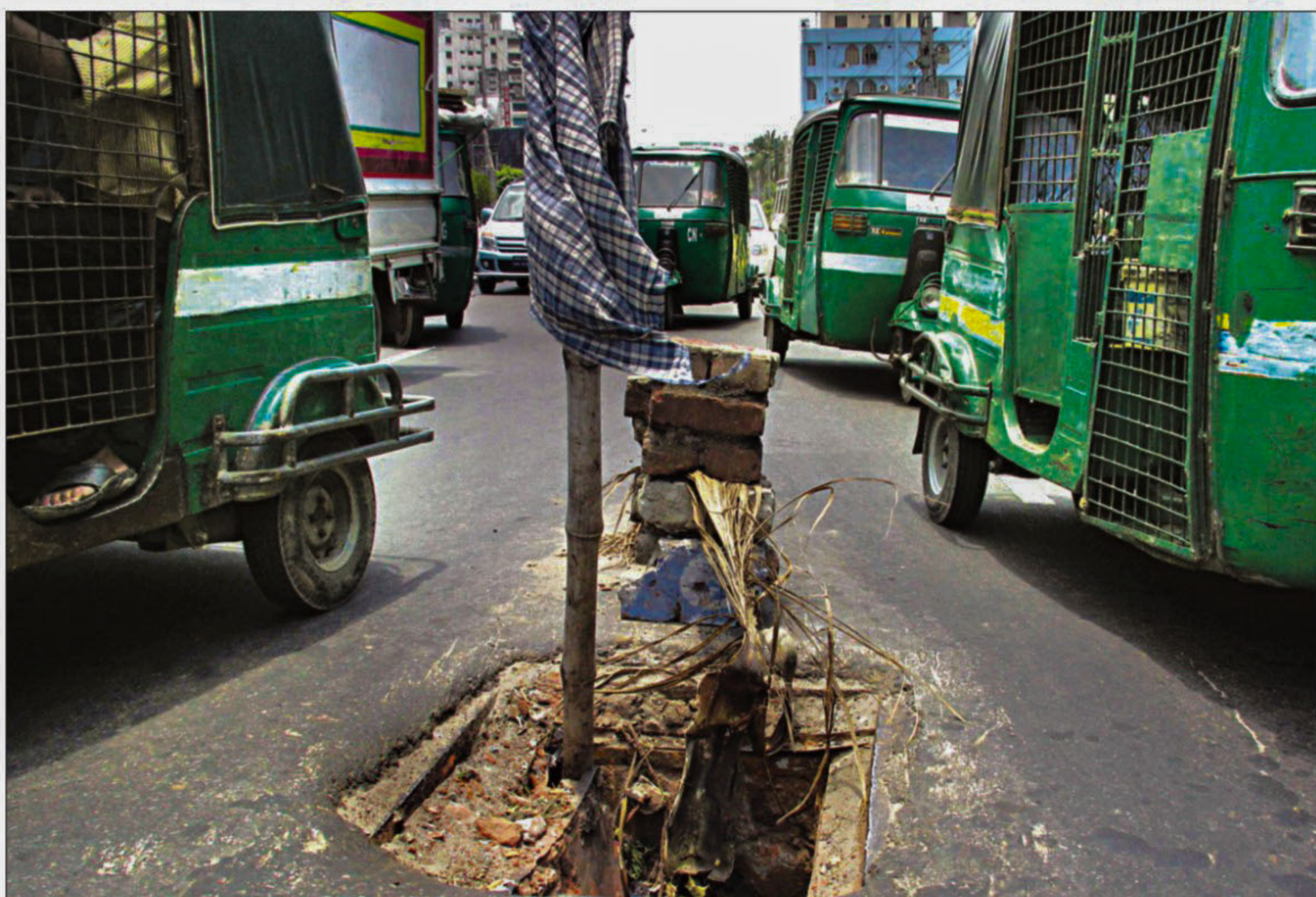
A manhole without cover in the middle of old airport road in the city poses danger to passengers, but the authorities concerned remain indifferent. Local people put up a bamboo pole to warn motorists of the danger. The photo was taken yesterday.
