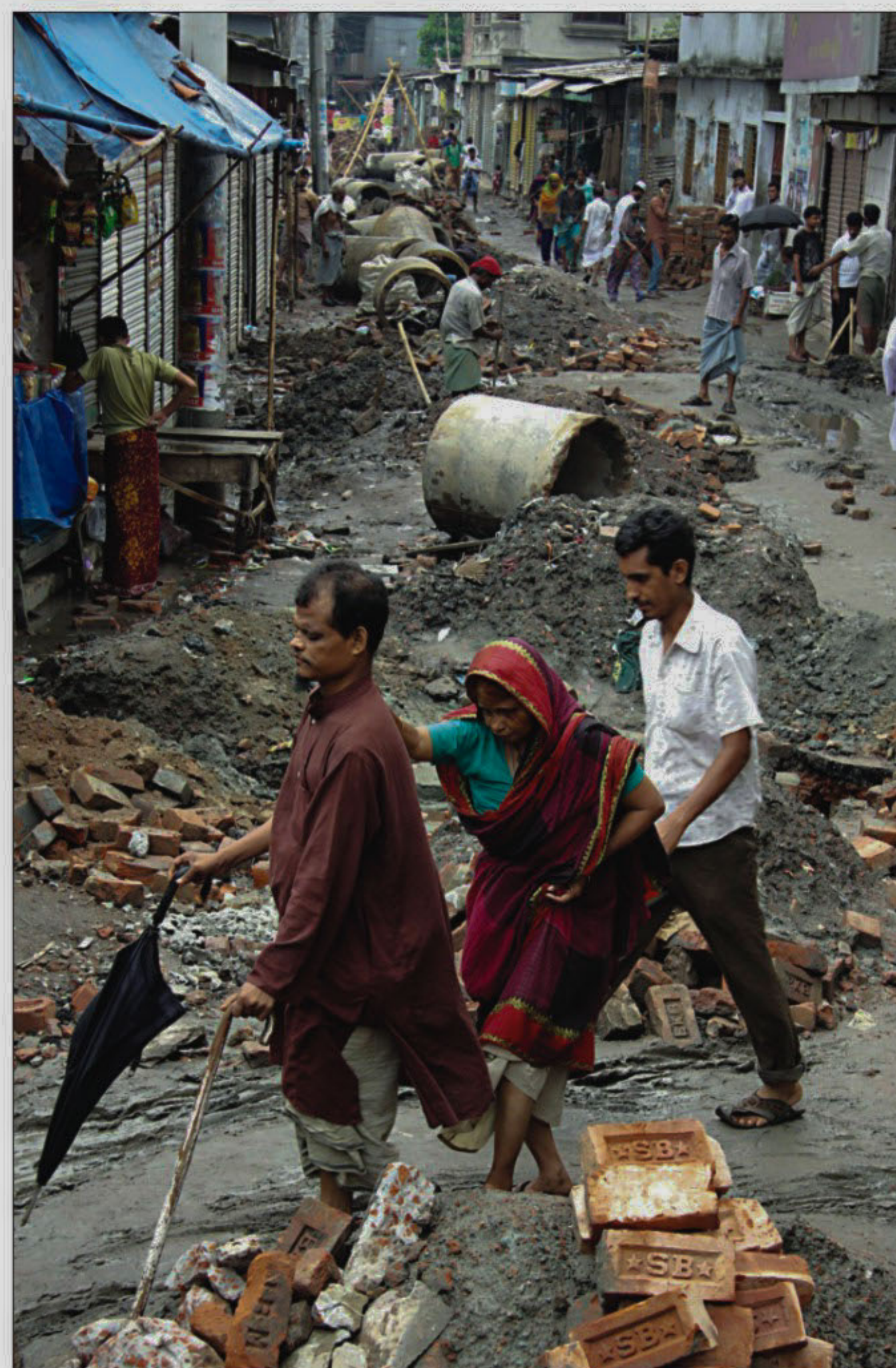
Work of installation of sewer lines at Lalbagh in the city is going on for a long time, causing suffering to pedestrians as well as local residents.
