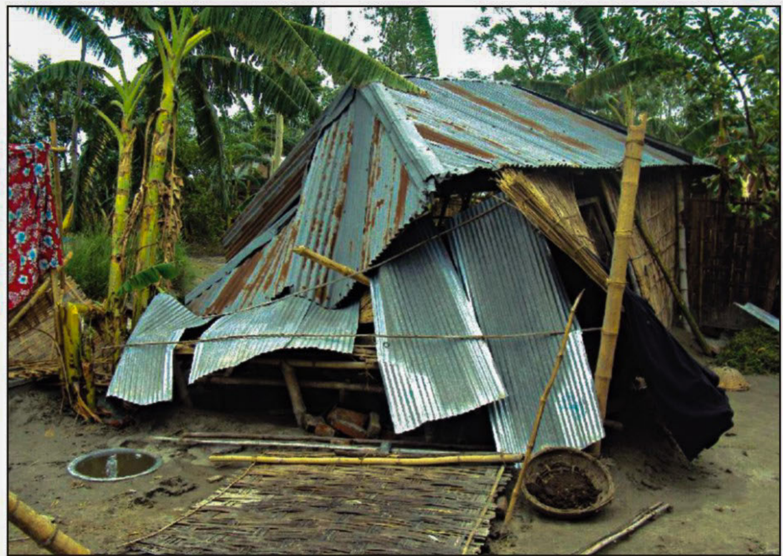
Nor'wester lashes 20 villages in different upazilas of Lalmonirhat districts early yesterday, damaging over 1,000 thatched and tin-roofed houses and injuring at least 10 people. Photo shows a damaged house at Mohishkhocho village under Aditmari upazila.
