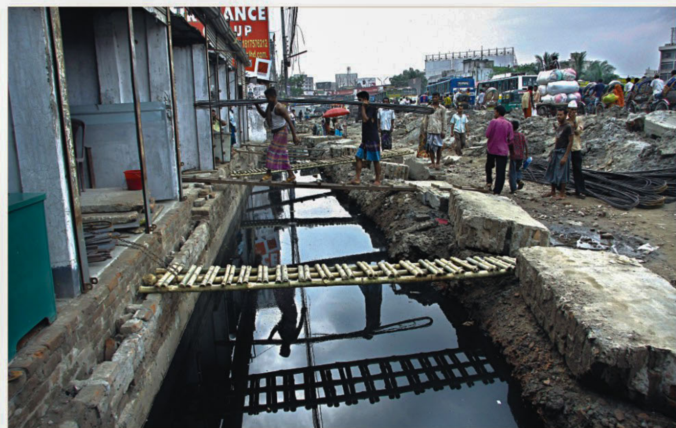
Dug up Dhaka-Chittagong highway at the capital's Jatrabari area. The highway was excavated about a month ago to lay sewer pipes. No progress in the work has been made since then. The photo was taken a few days ago.
