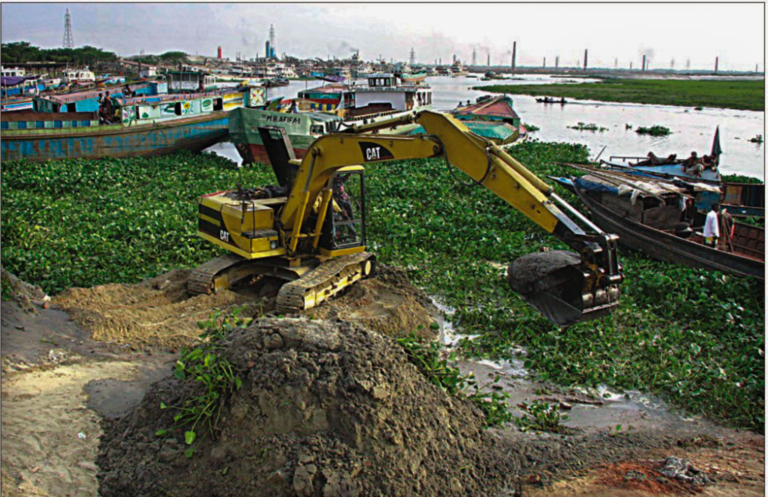
A BIWTA excavator removes soil from an encroached upon section of the river Turag near Gabtali yesterday. But the agency dumps it right on the bank making it easily available for anyone wanting to fill up the river again. The carelessness renders the entire exercise futile. PHOTO: SK ENAMUL HAQ
