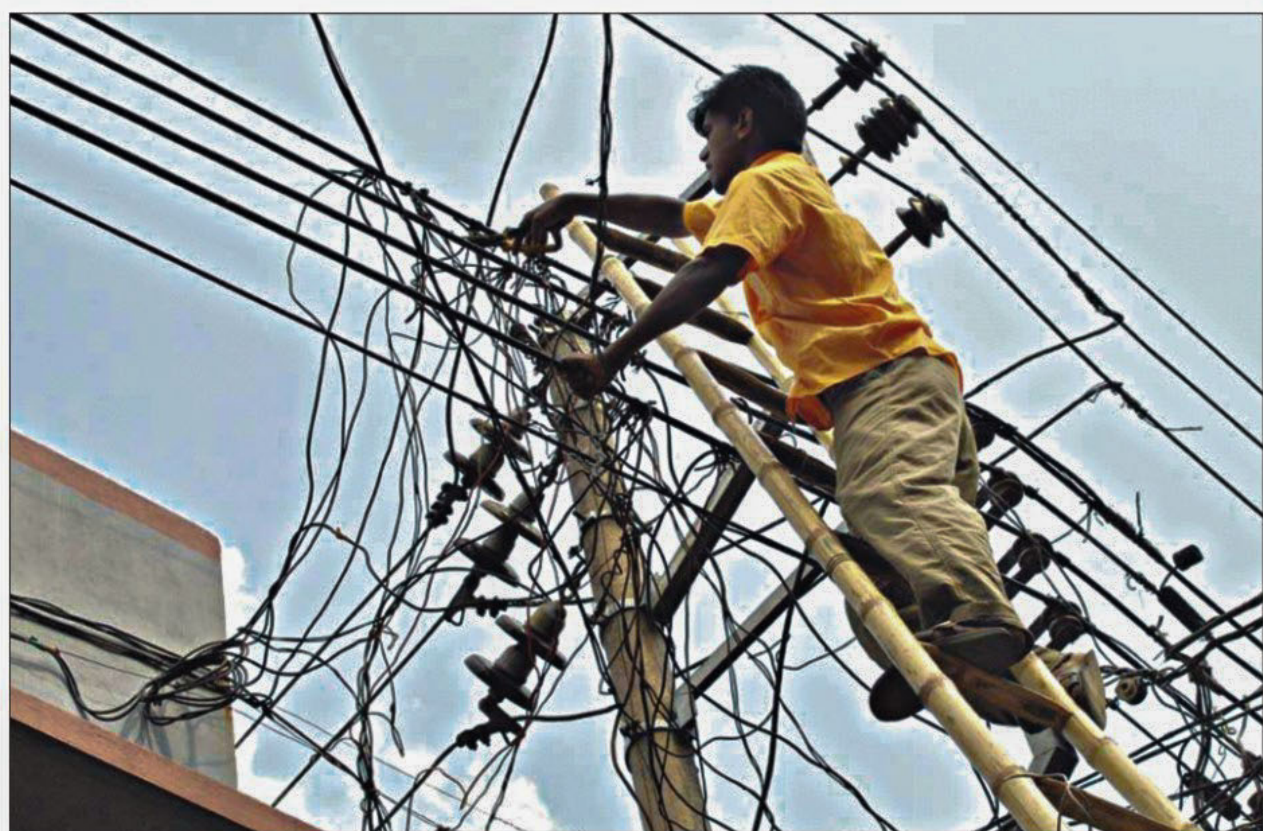
A team of DPDC and a mobile court snaps electricity connections during a drive against illegal connections and bill defaulters in the city's Bashabo, Nondipara, Madartek and Goran areas yesterday.
