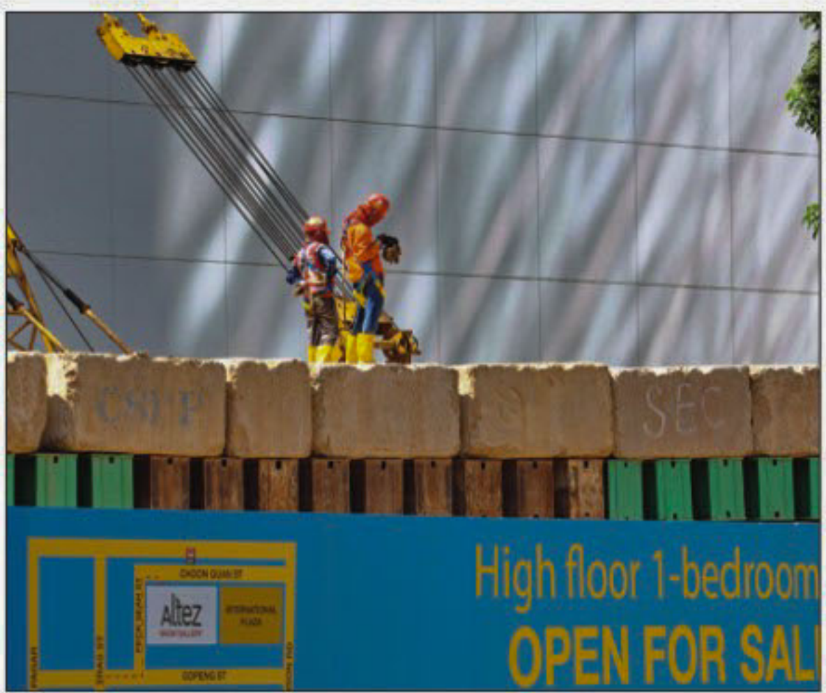
Workers stand on concrete slabs where a high floor apartment and office building are being constructed in Singapore yesterday. Singapore's housing sector is still sizzling despite government measures to cool it down, with demand fuelled by a strong economy and foreign investor confidence.
