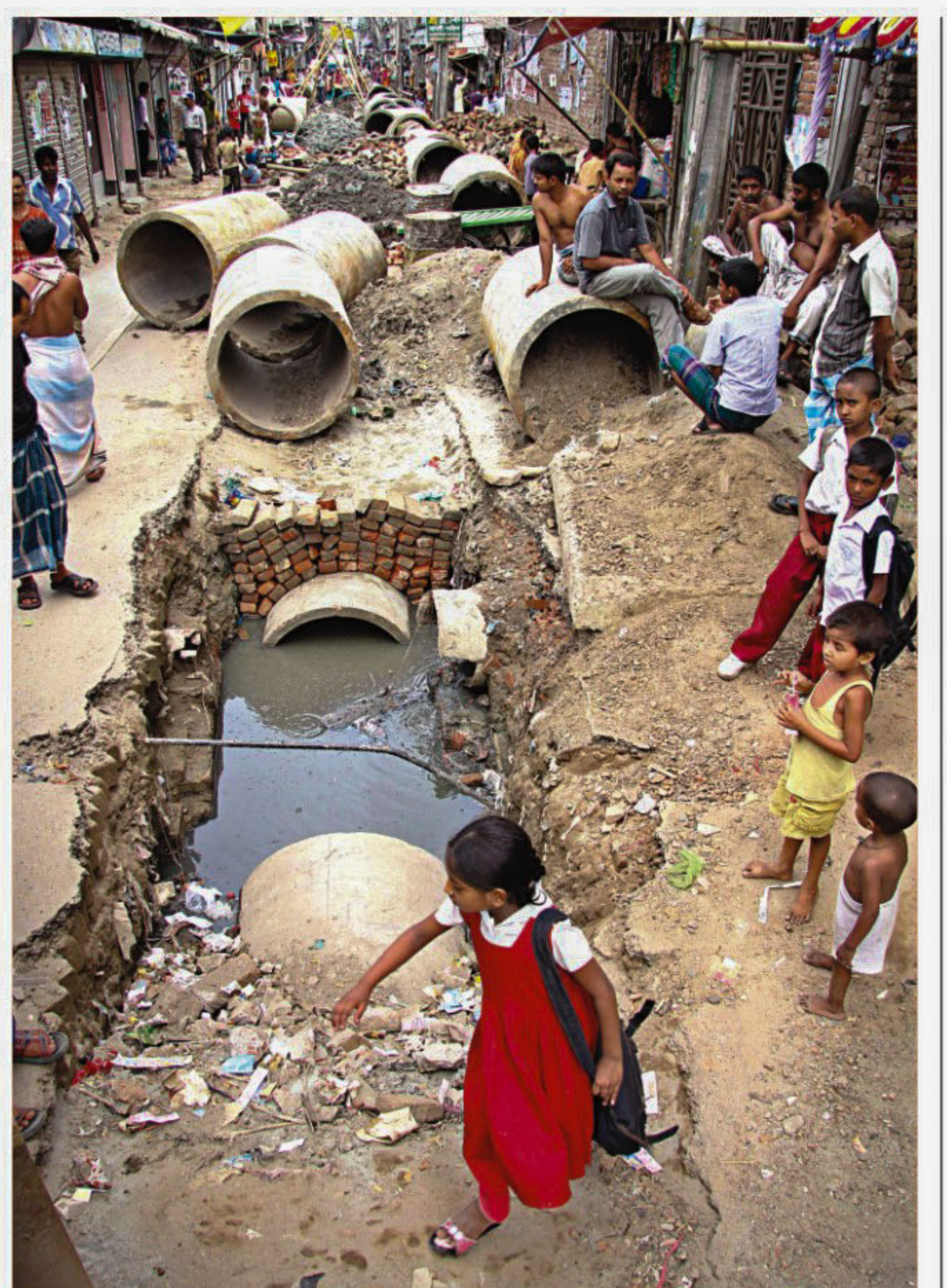
Dug up JN Saha Road in the capital's Lalbagh area for laying sewer pipes. Locals fear the sewer will be dysfunctional soon after the work completes, as they allege the contractor has been using low quality materials. The photo was taken yesterday. PHOTO: ANISUR RAHMAN
