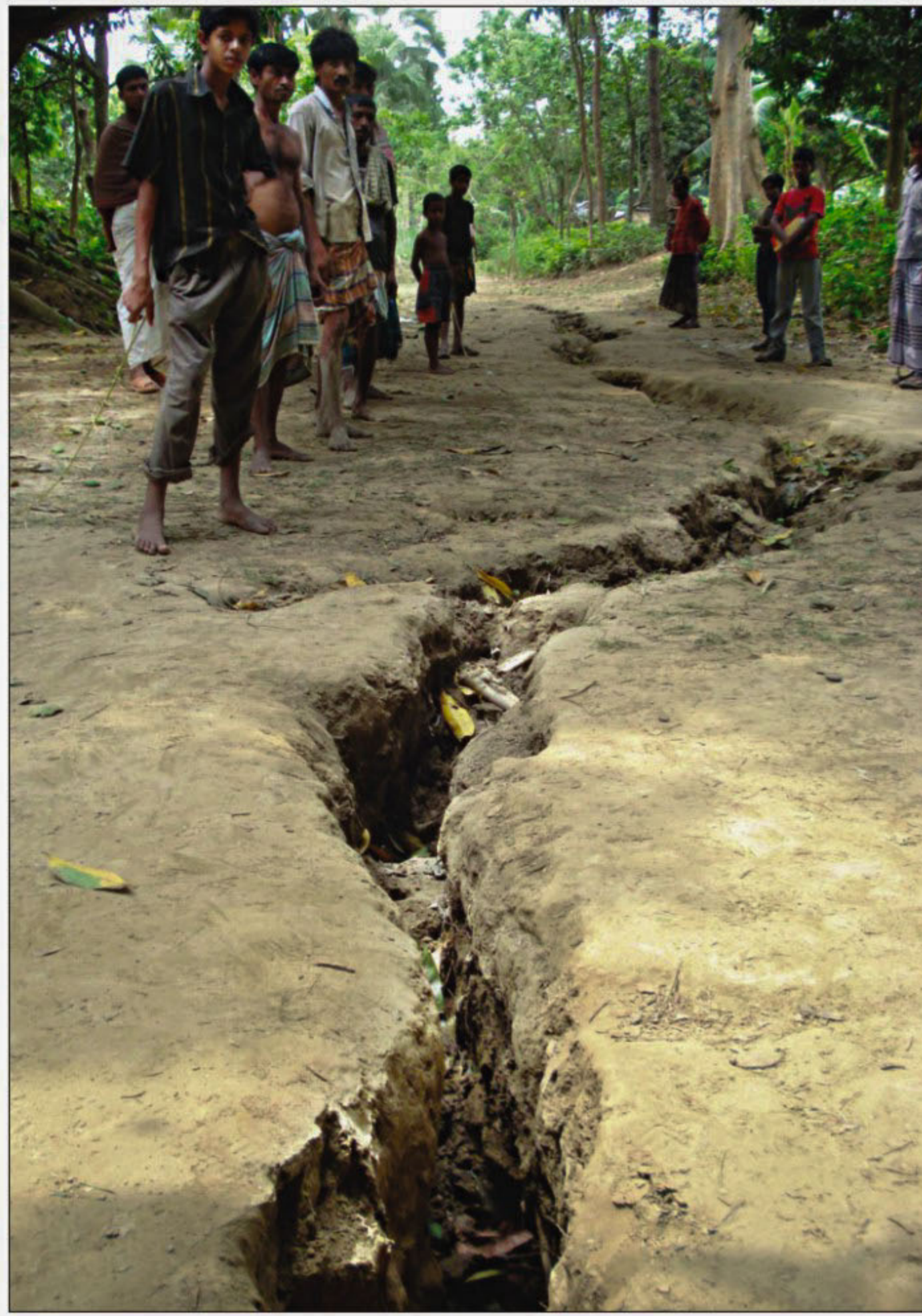
A 300-metre-long crack has developed at Nawpara village under Mohanpur upazila of Rajshahi. According to the villagers, the crack is getting longer and deeper.
