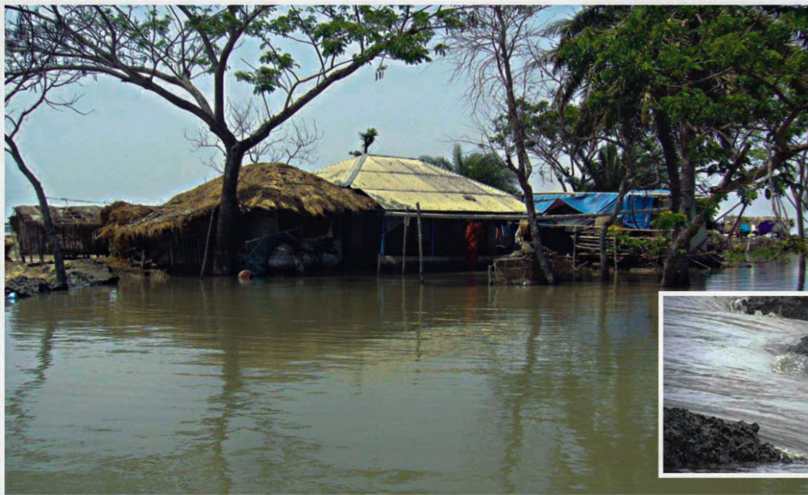
Jaliakhali village of Kamarkhola union in Khulna has submerged again as the dike collapsed in the massive pressure of river water recently. Inset, the broken segment of the embankment. The sufferings of these Aila-hit people appear to be never ending.
