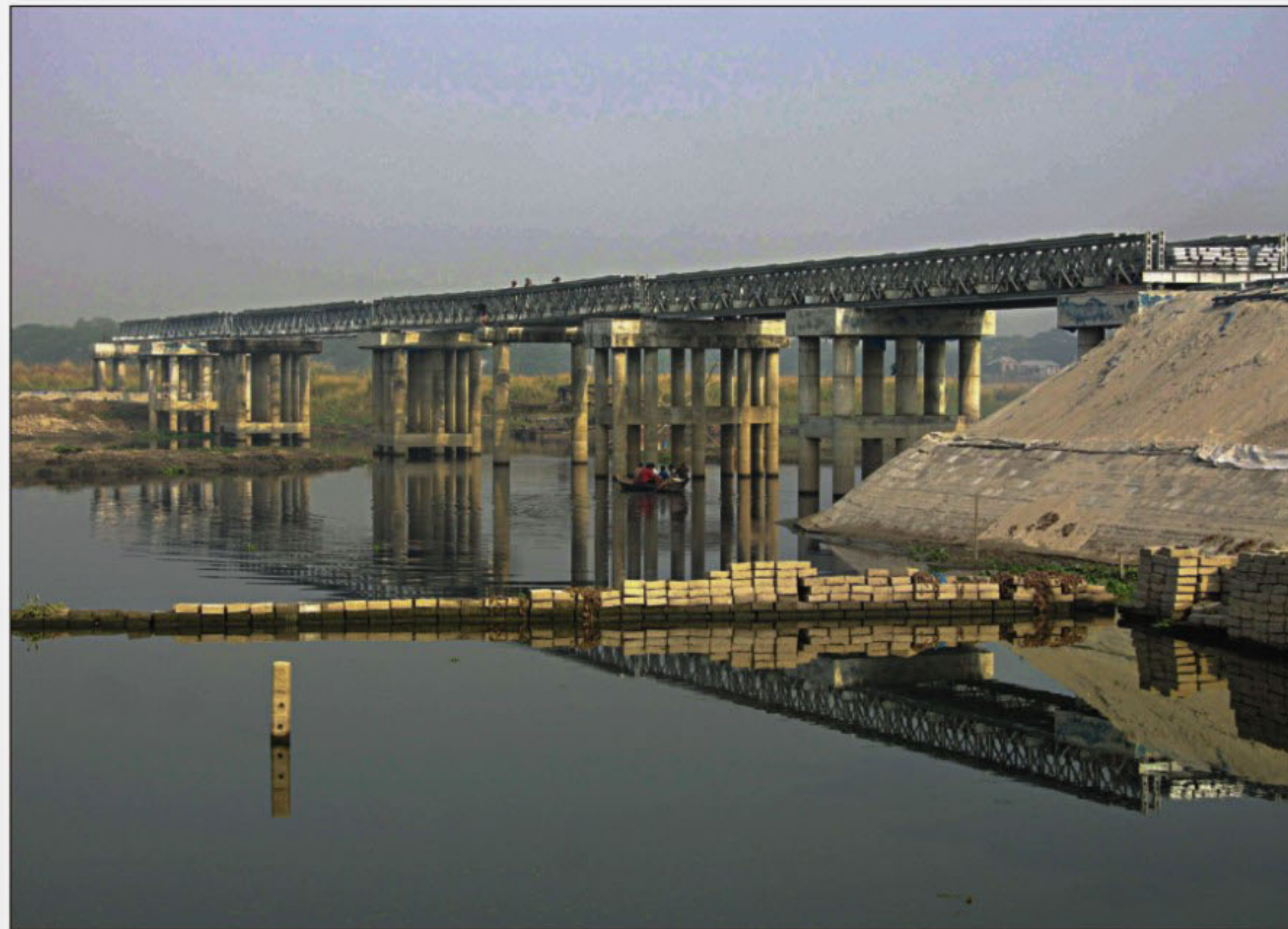
The photo taken in November shows the Pratyasha Bridge (Nolnichala Bailey Bridge) on the Turag in Ashulia. The taskforce for saving rivers has identified it as having poor clearance for vessels and will recommend its demolition and rebuilding. PHOTO: FILE
