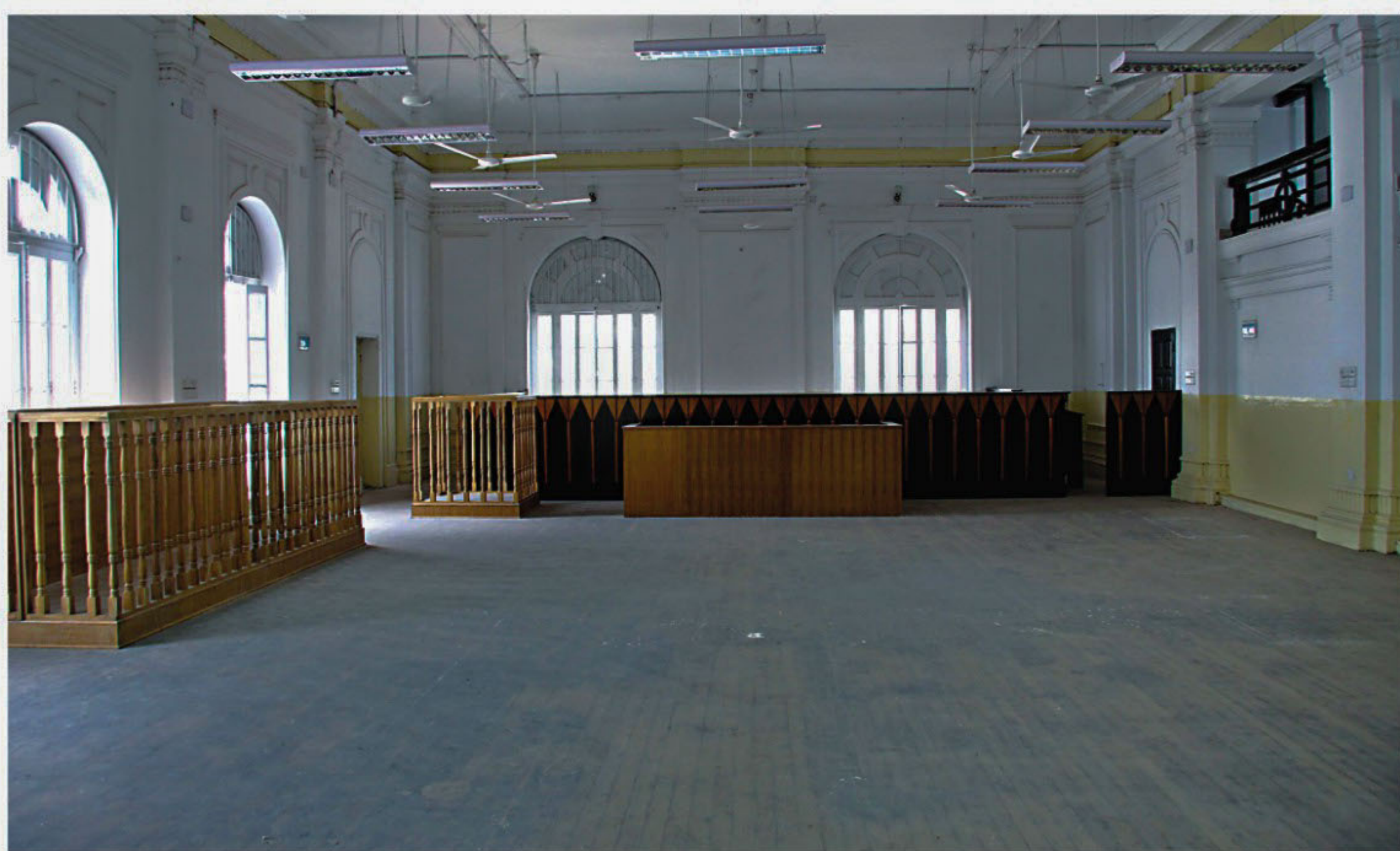
The courtroom for trying war criminals in the old High Court building is being renovated before the trial starts.
