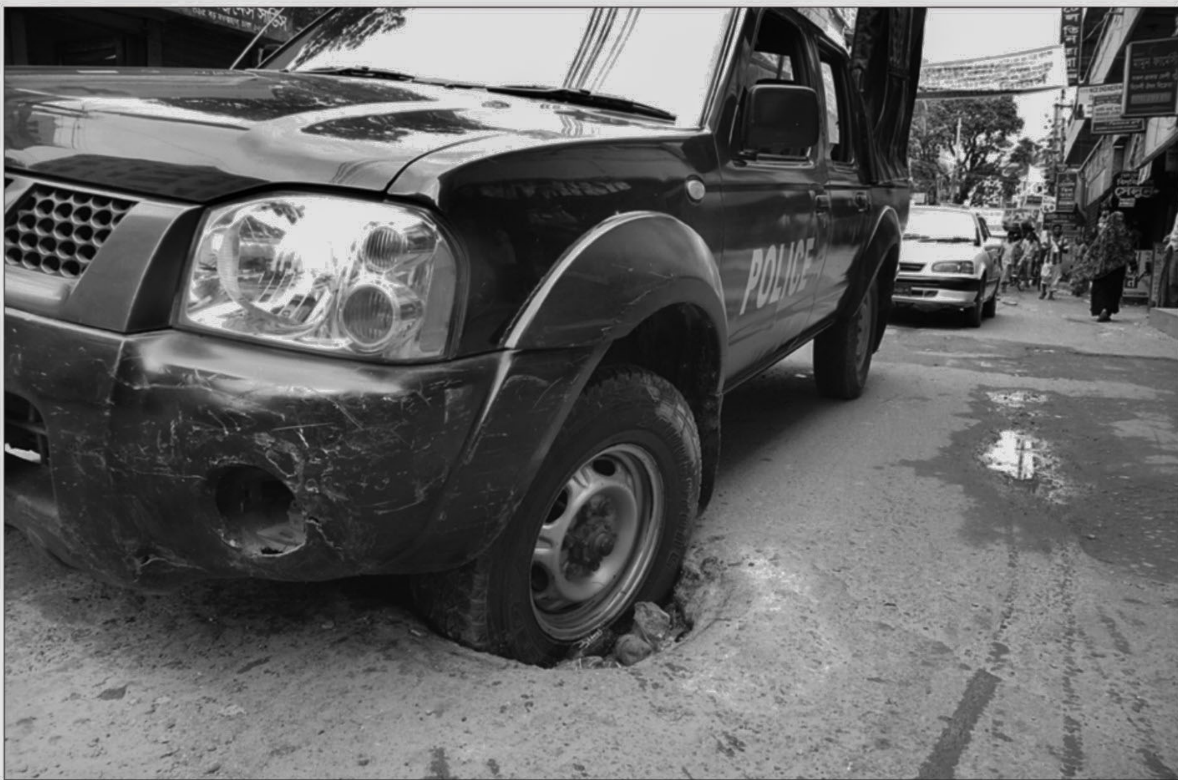
A wheel of a police van got stuck in a pothole near Maghbazar mosque in the city yesterday. Potholes have developed on many roads, hampering smooth movement of vehicles, but the authorities remain indifferent to the problem.
