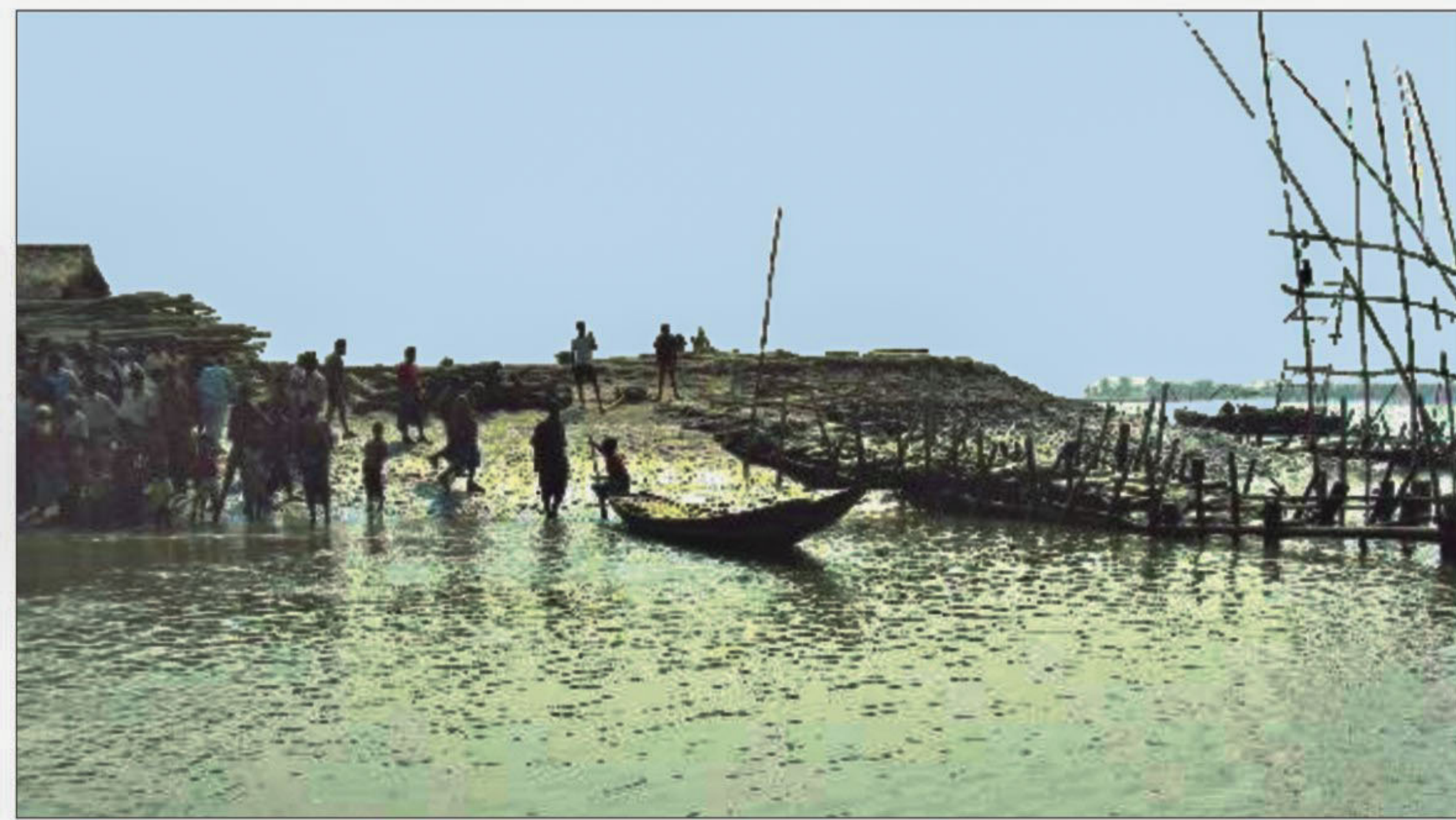
PHOTO: STAR Left without any repair since cyclone Aila hit the area on May 25 last year, this breached portion of embankment at Garkompur on Kobadak River in Padmapukur union of Shyamnagar upazila under Satkhira district leaves locals vulnerable to added sufferings during the coming monsoon. A few other large breaches including those at Jhhapa in the same union and Chakbara on the Kholetua River in Gabura union of Shyamnagar upazila are also in the same condition.
