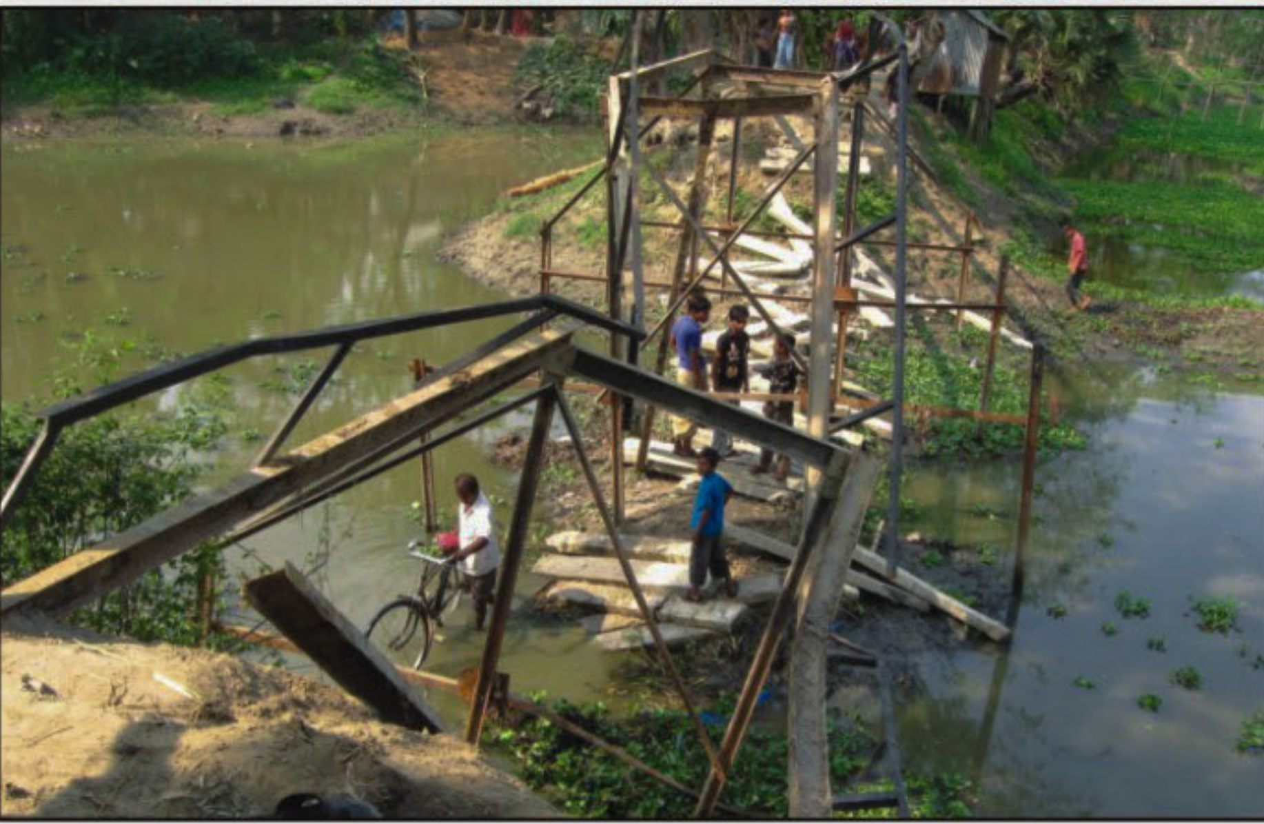
PHOTO: STAR This bridge at Mohishmari village on Tekerhat-Mohishmari road in Rajoir upazila under Madaripur district collapsed when around 30 children were crossing it on their way to home from a local madrasa yesterday. With average to serious injuries, 12 of the children were admitted to Rajoir and Tekerhat hospitals while others sustained minor injuries.
