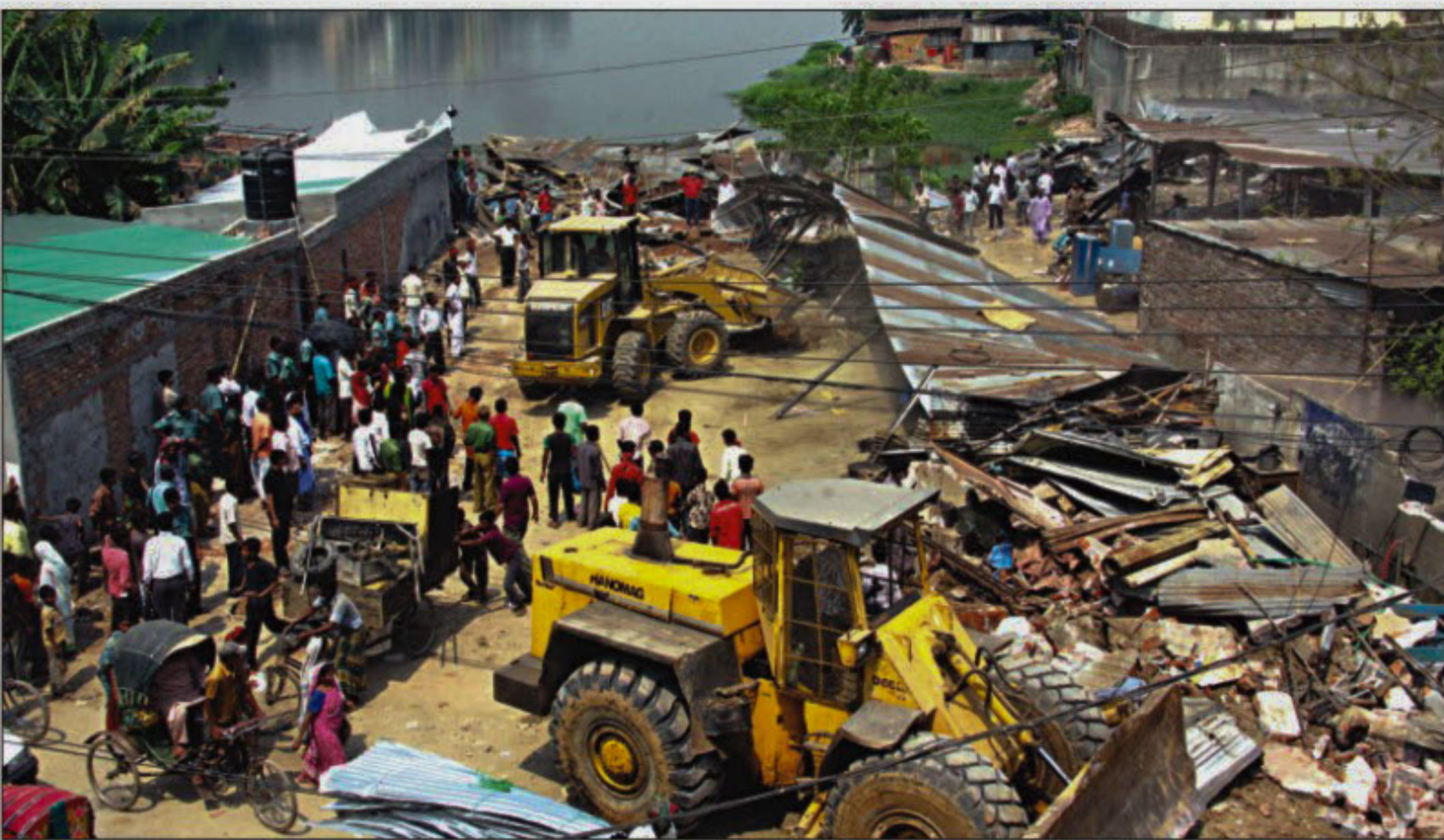
Rajuk knocks down small structures occupying Gulshan Lake along Gulshan-South Badda Link Road yesterday. Most of these dwellings belonged to poor people. However, the authorities could not tear down buildings owned by big fishes due to court orders.
