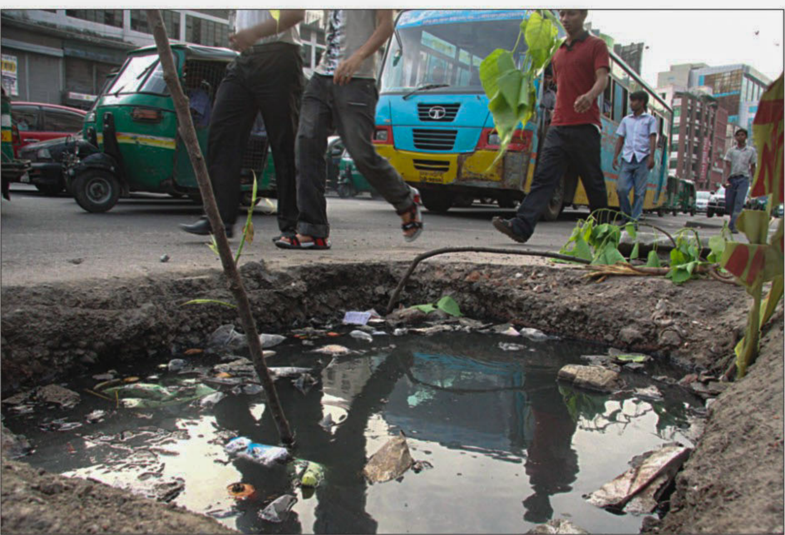
A big pothole develops on the Kazi Nazrul Islam Avenue at Karwan Bazar in the city. Speeding vehicles often fall into the hole, but the authorities appear to be indifferent to the problem. The photo was taken yesterday.
