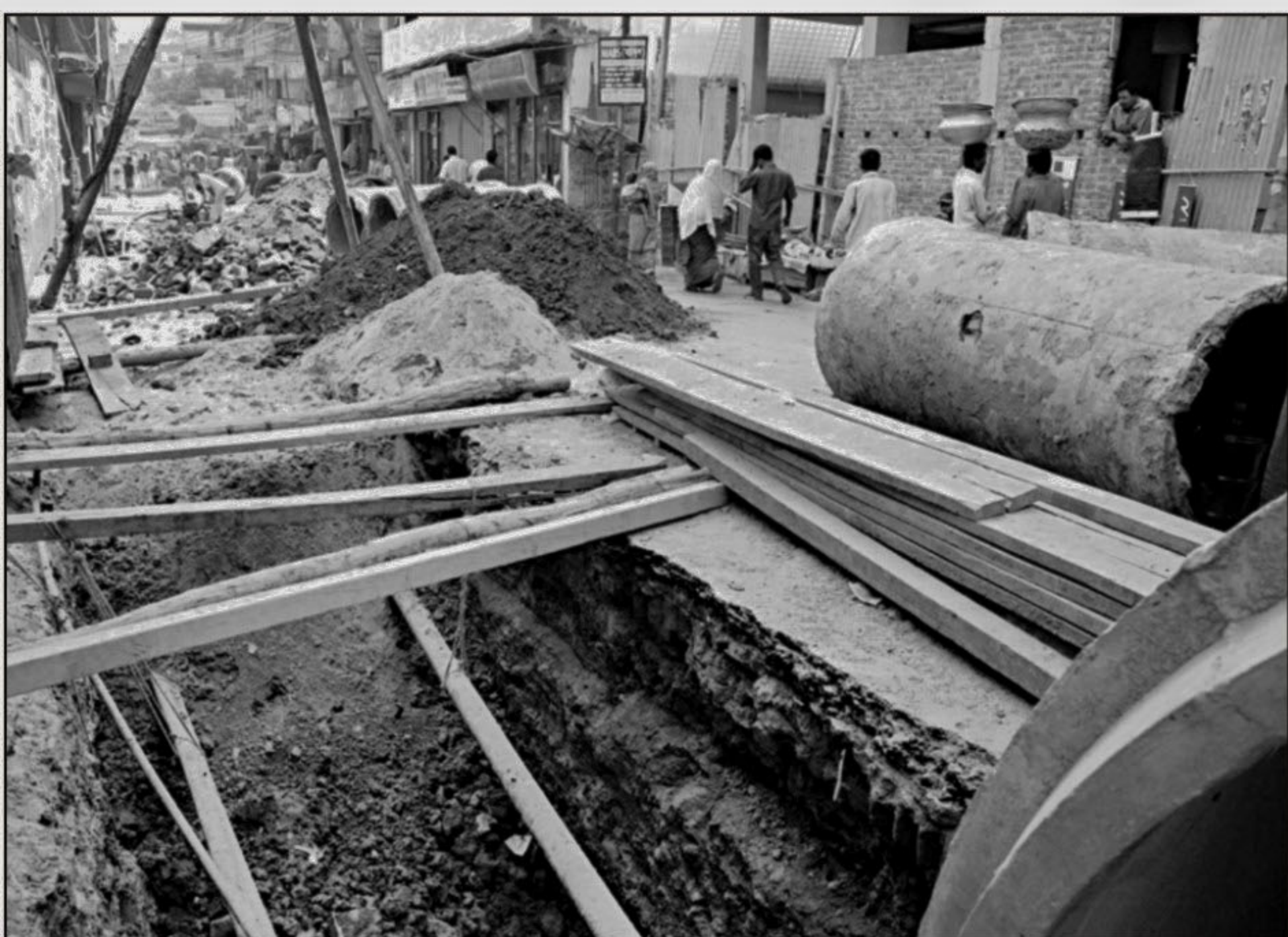
Dhaka Wasa workers dig in the middle of Gopibagh RK Mission road to instal sewer pipes almost a month ago, but slow work has been causing suffering to pedestrians and local residents. The photo was taken yesterday.
