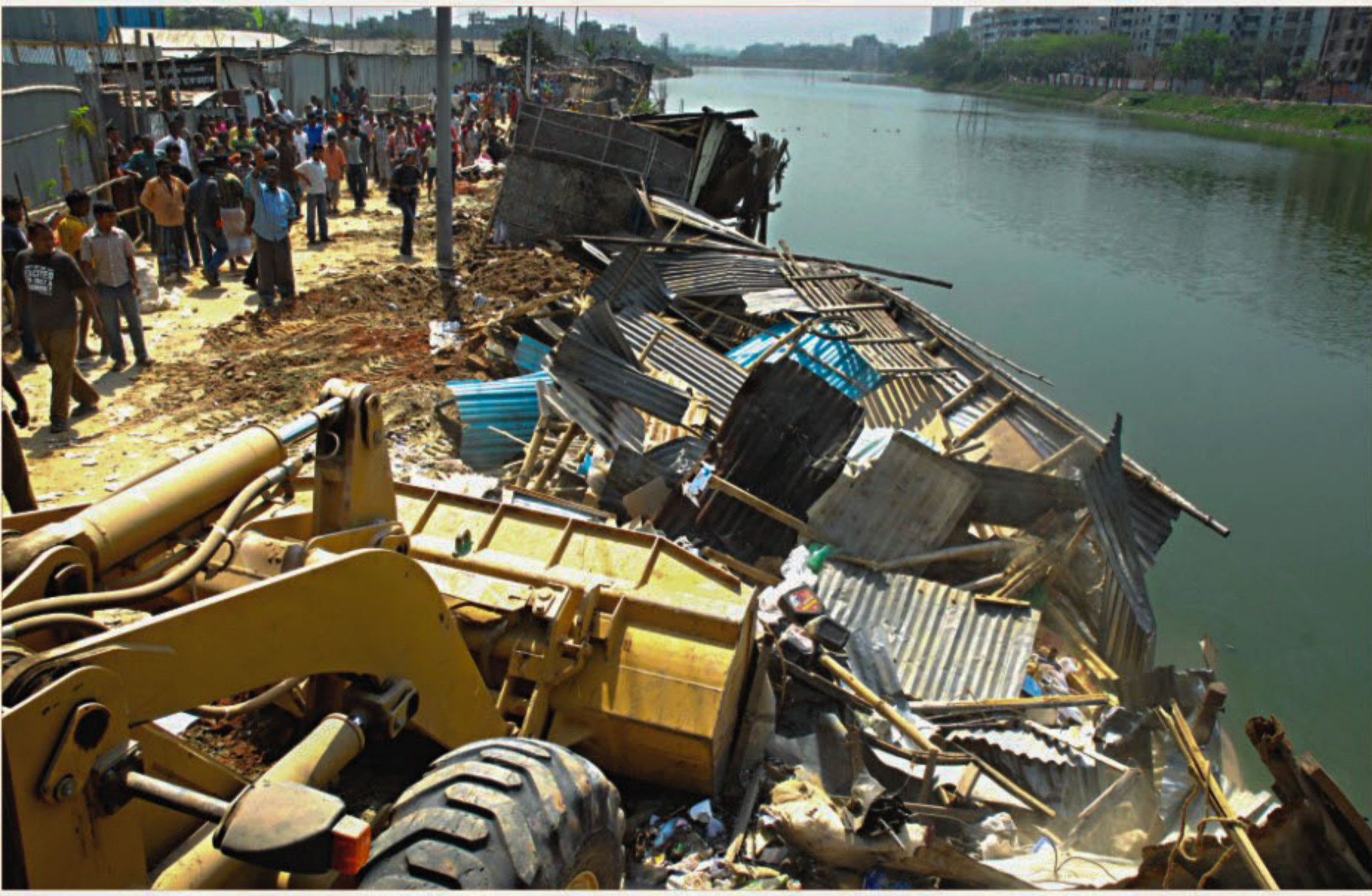
Rajdhani Unnayan Kartripakkha in presence of police and Rajuk officials demolishes around 100 illegal structures on Gulshan Lake at city's Shahjapur yesterday. Gulshan Lake was declared ecologically critical in 1997. The High Court directed the government to free the lake from encroachments by August 31 this year.
