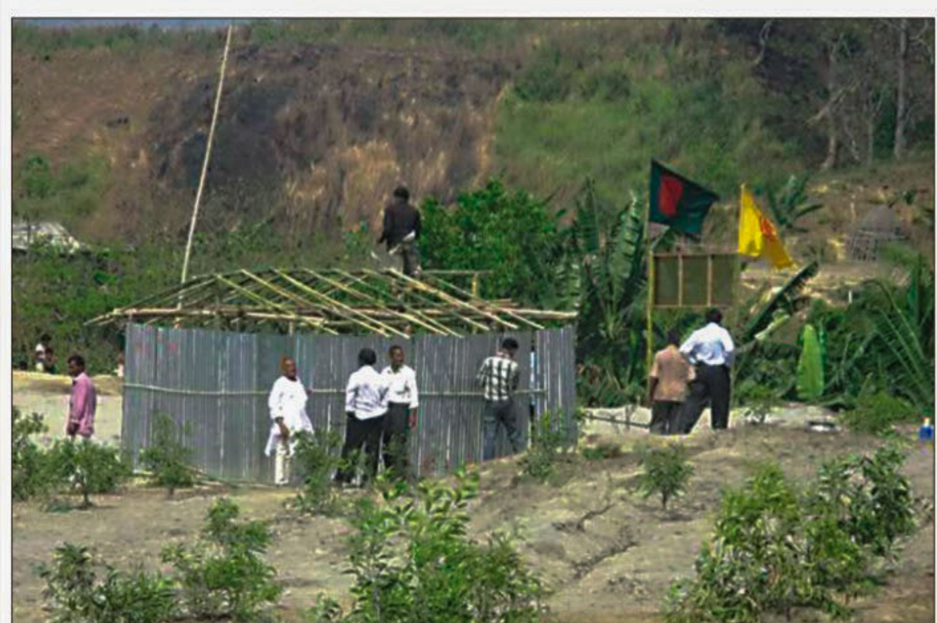
A group of people with a made-up banner "Bangladesh Freedom Fighters' Rehabilitation Society" build houses flattening a hill at Kolatoli in Cox's Bazar. They also hoisted the national flag and the flag of Bangladesh Muktiyoddha Sangsad despite local Bangladesh Muktiyoddha Sangsad leaders' request not to use their flags for destroying the hills.
