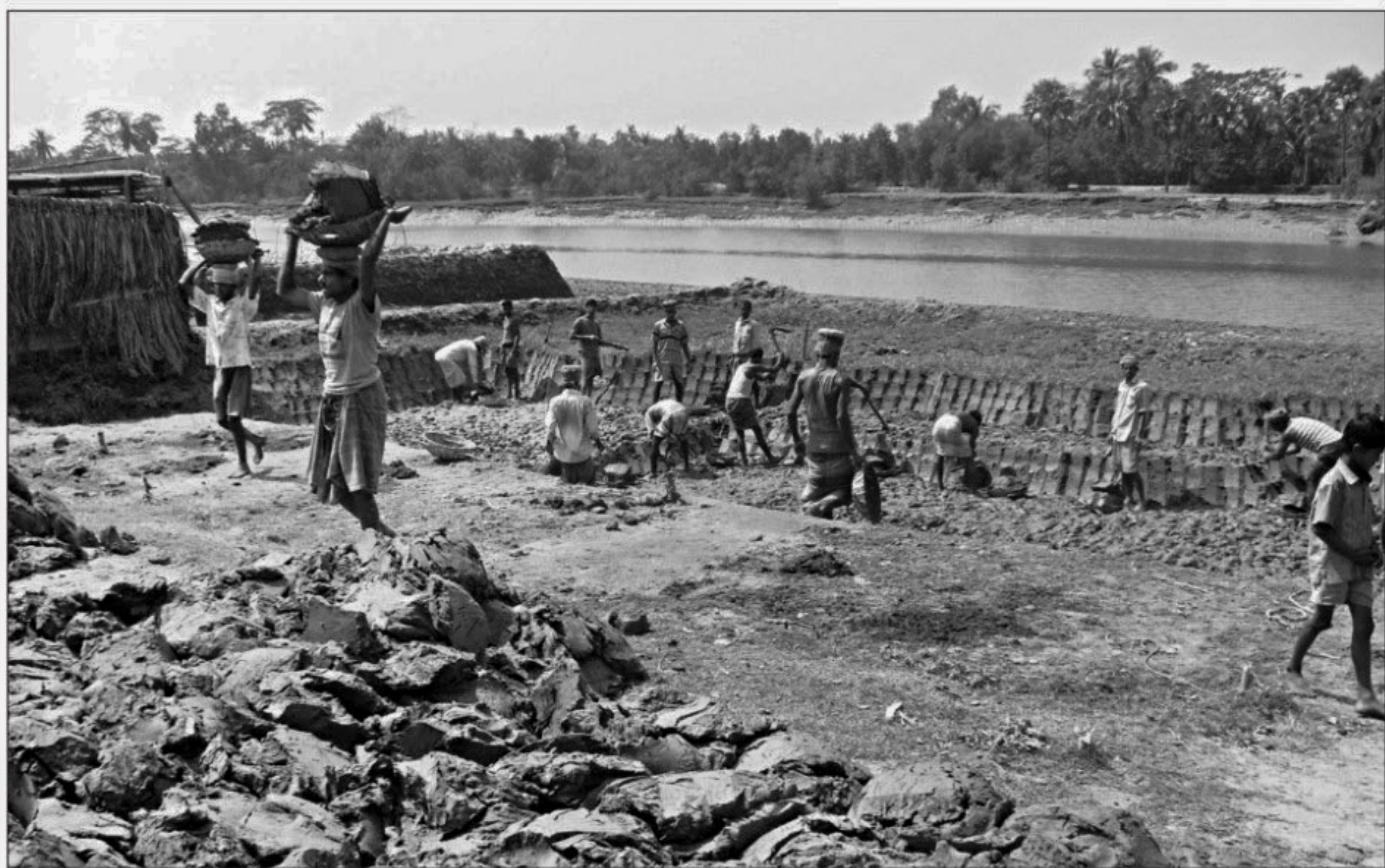
Labourers working under a project at Khegraghat cluster village in Dema union of Bagerhat district. The government has taken 85 such projects to provide employment opportunity to a large number of destitute and landless people in 66 upazilas of 41 districts.
