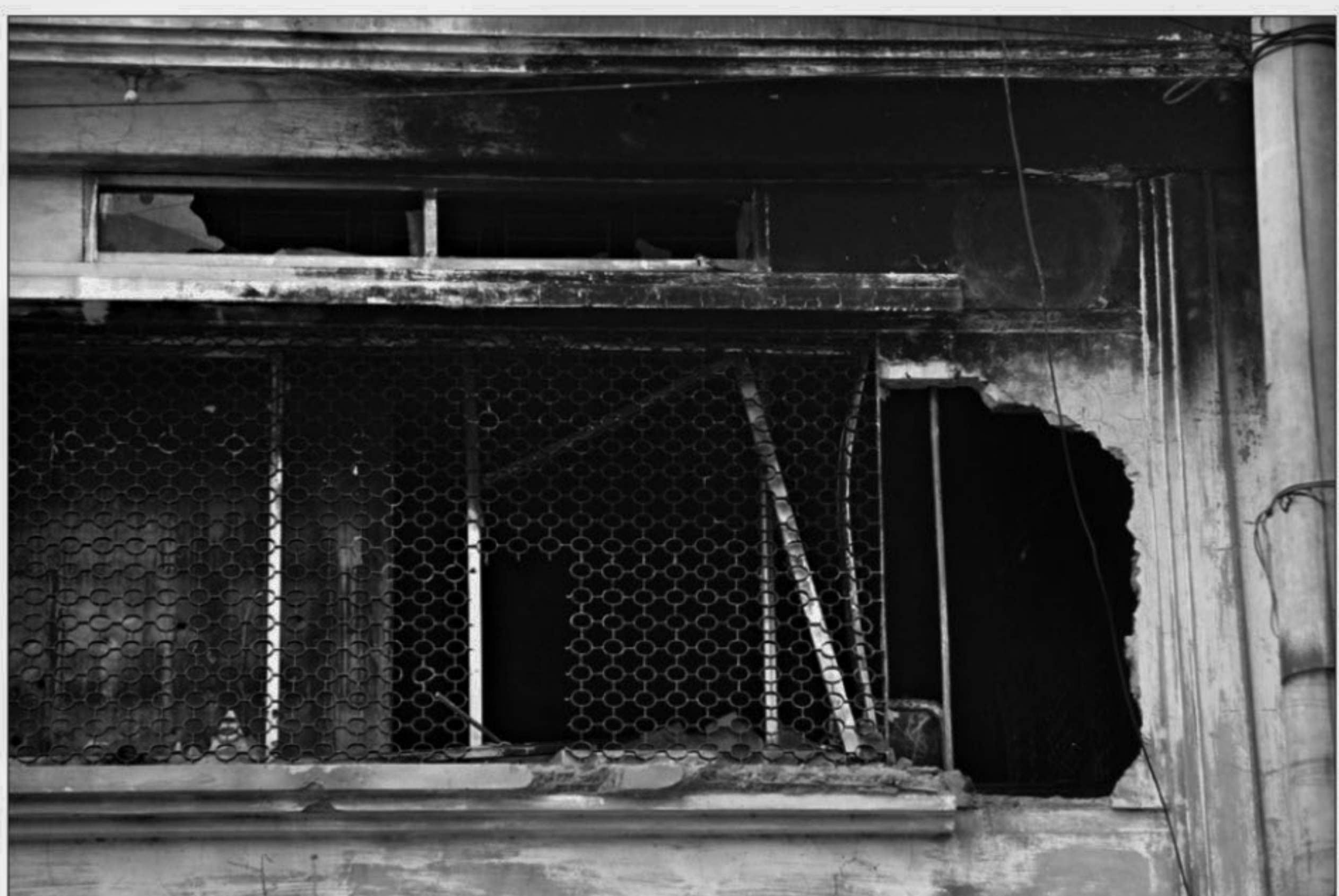
Fire service personnel had to break portion of Garib and Garib factory wall to rescue workers.
