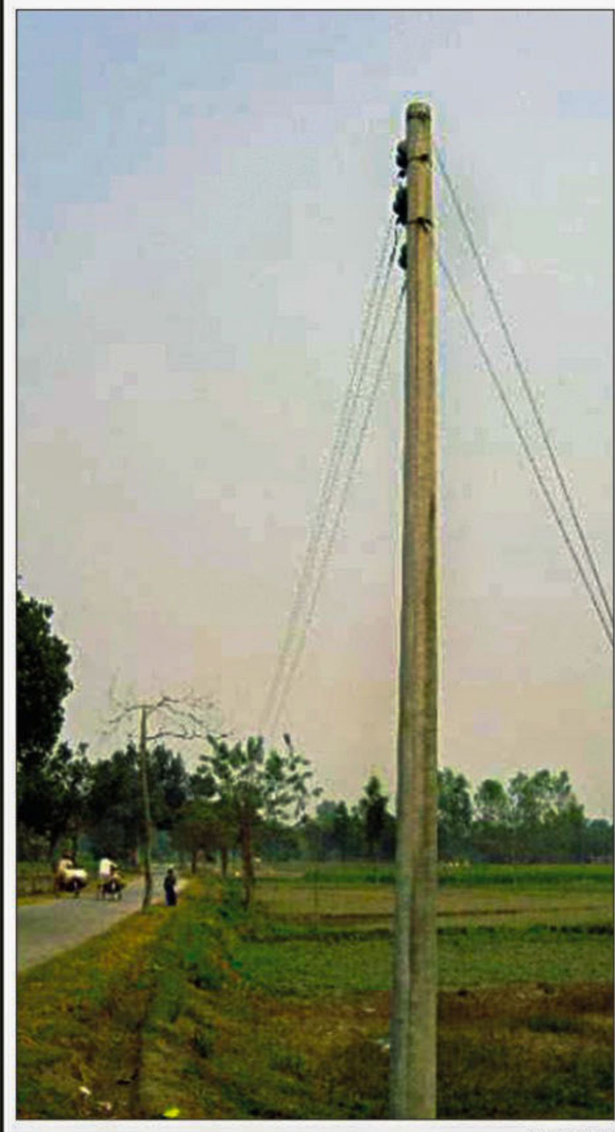
Setting up of electricity poles and cables continues as authorities started work on Monday to supply power to Dahagram-Angarpota enclave.
