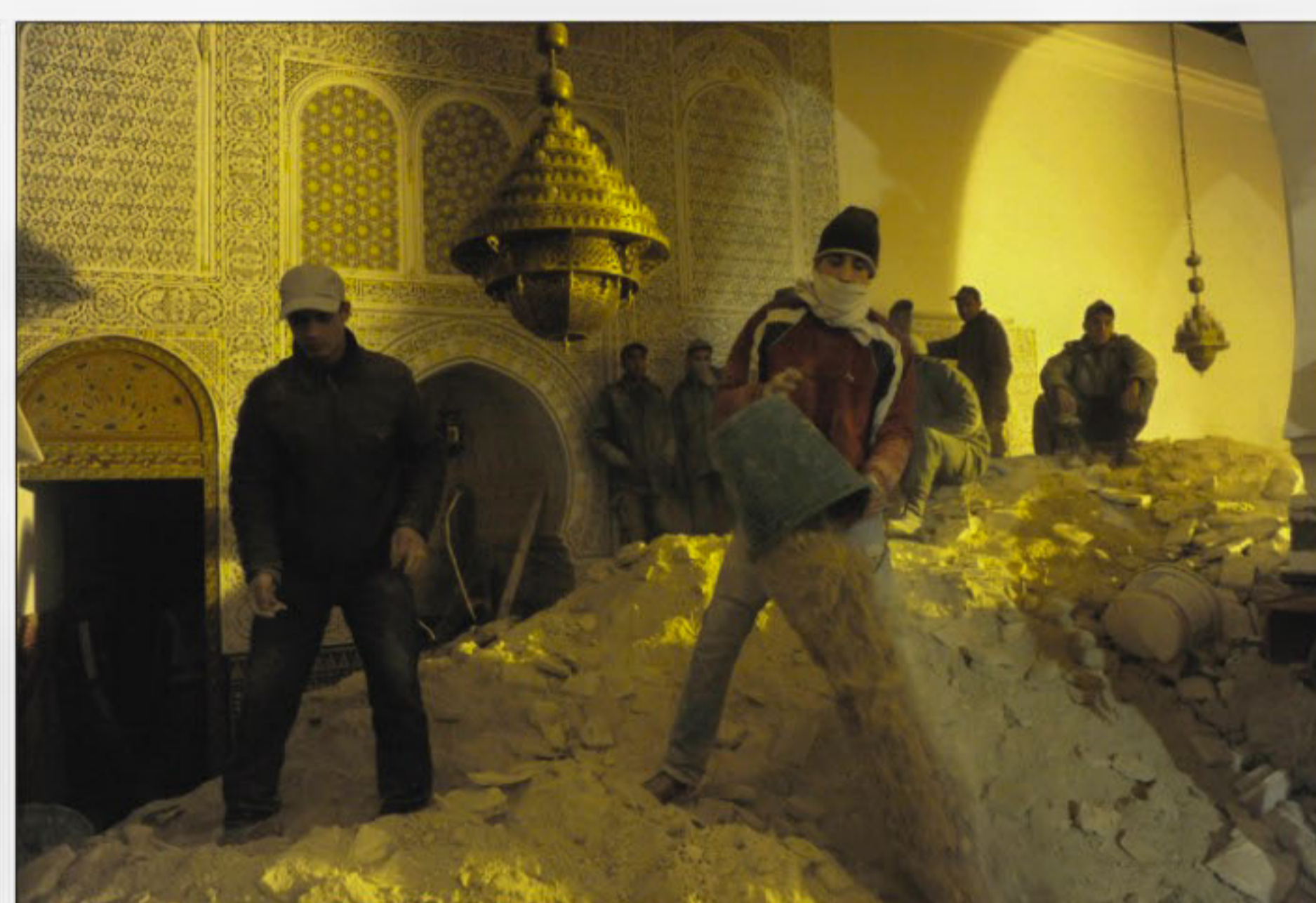
Moroccan volunteers of the 'Medina' help rescue workers to look for survivors and bodies after the minaret of a mosque collapsed during Juma prayers in Morocco's central town of Meknes on Friday killing 41 people and injuring 71 others. The collapse came after "heavy rains which lashed the region for several days," a television report said.
