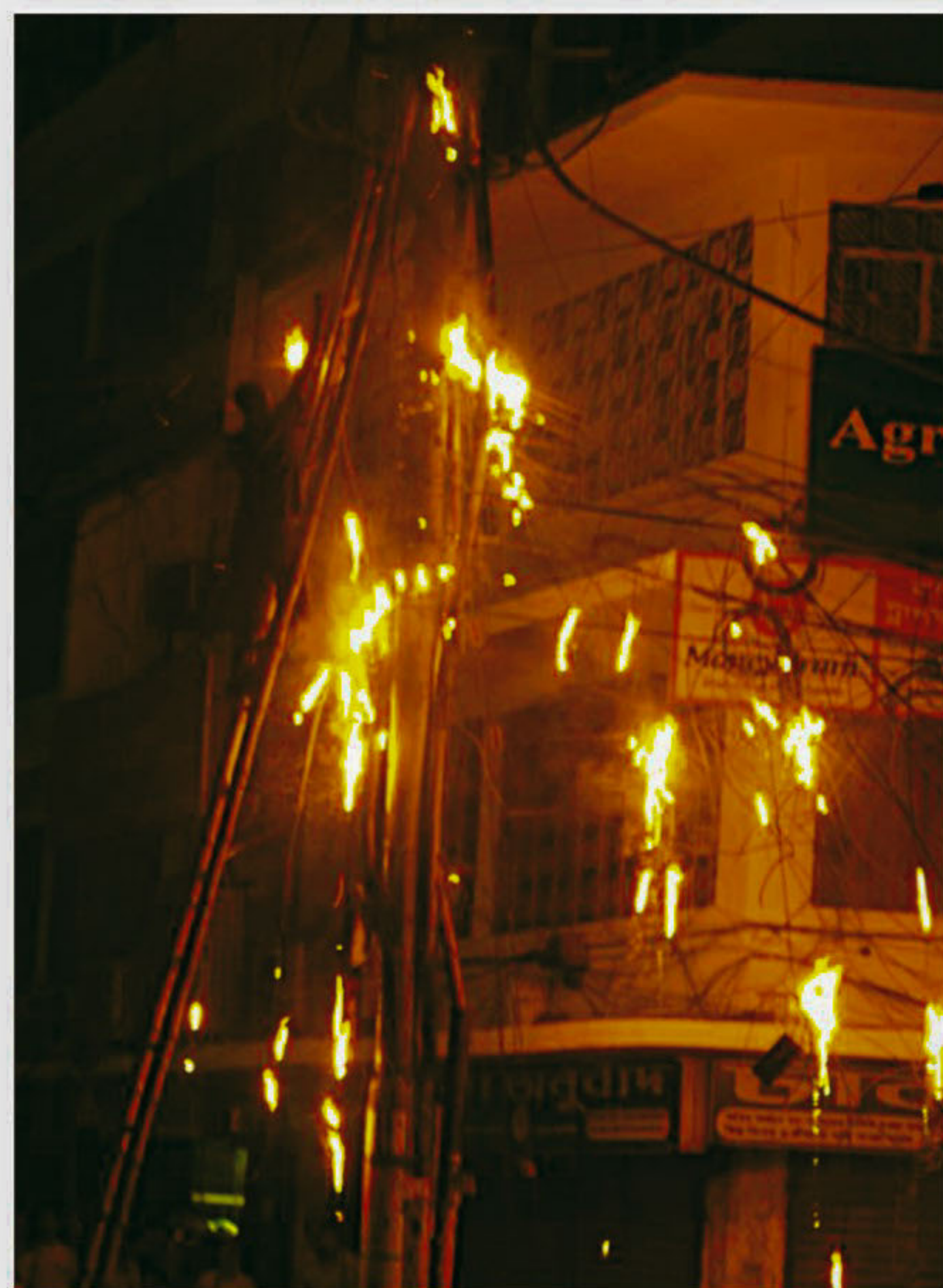
Overhead cables catch fire following an electrical short-circuit at a transformer at Dainik Bangla intersection in the city yesterday evening, damaging electrical and Internet cables.
