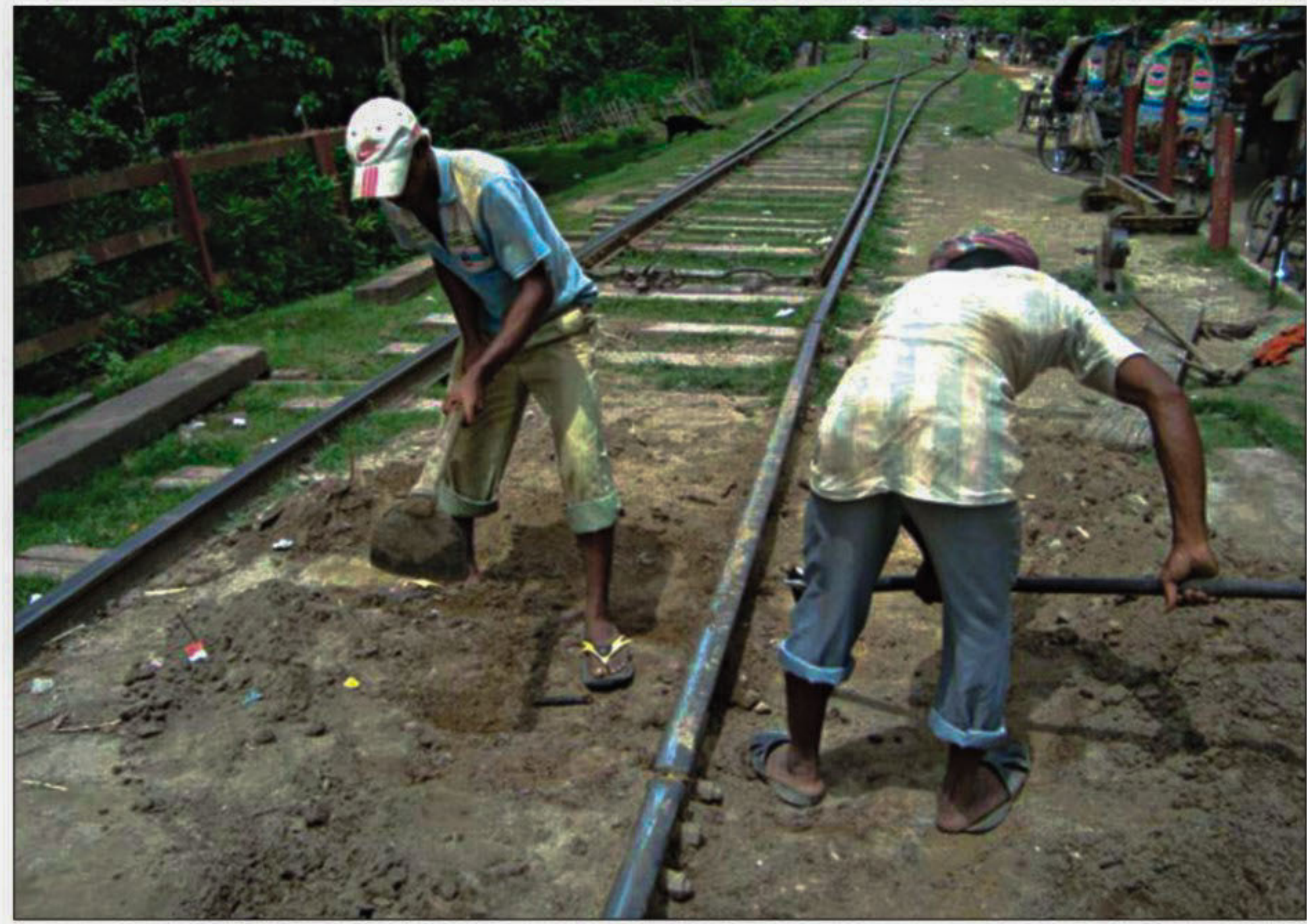
Two labourers are seen repairing rail lines near the outer signal of Chapainawabganj railway station recently as the tracks, laid without any stone chips, have turned risky for trains. PHOTO: STAR
