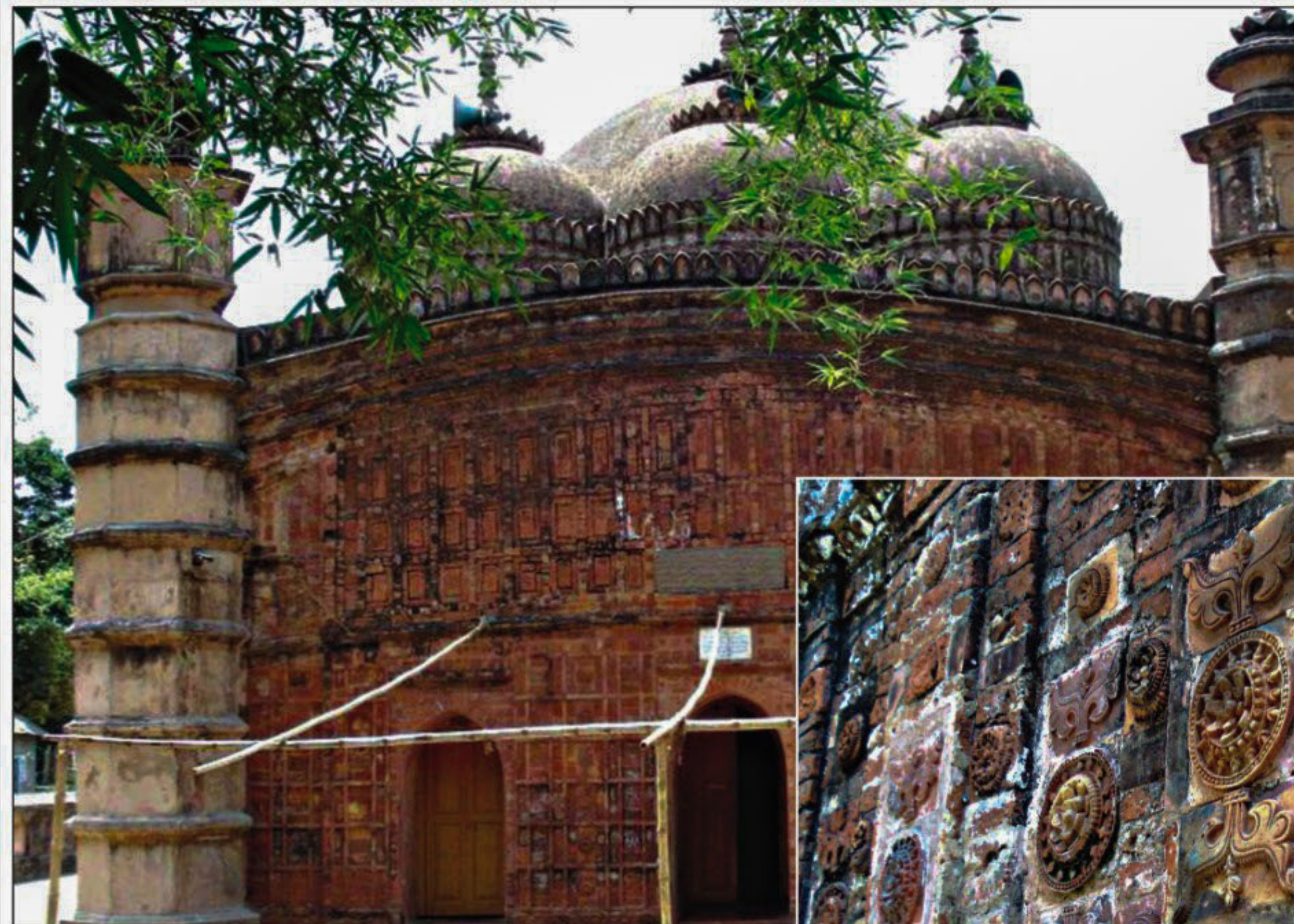
Four century-old Atia Mosque in Delduar upazila of Tangail still remains an impressive structure. Inset, artistic terracotta decorations of the beautiful mosque are decaying due to lack of proper maintenance. PHOTO: STAR
