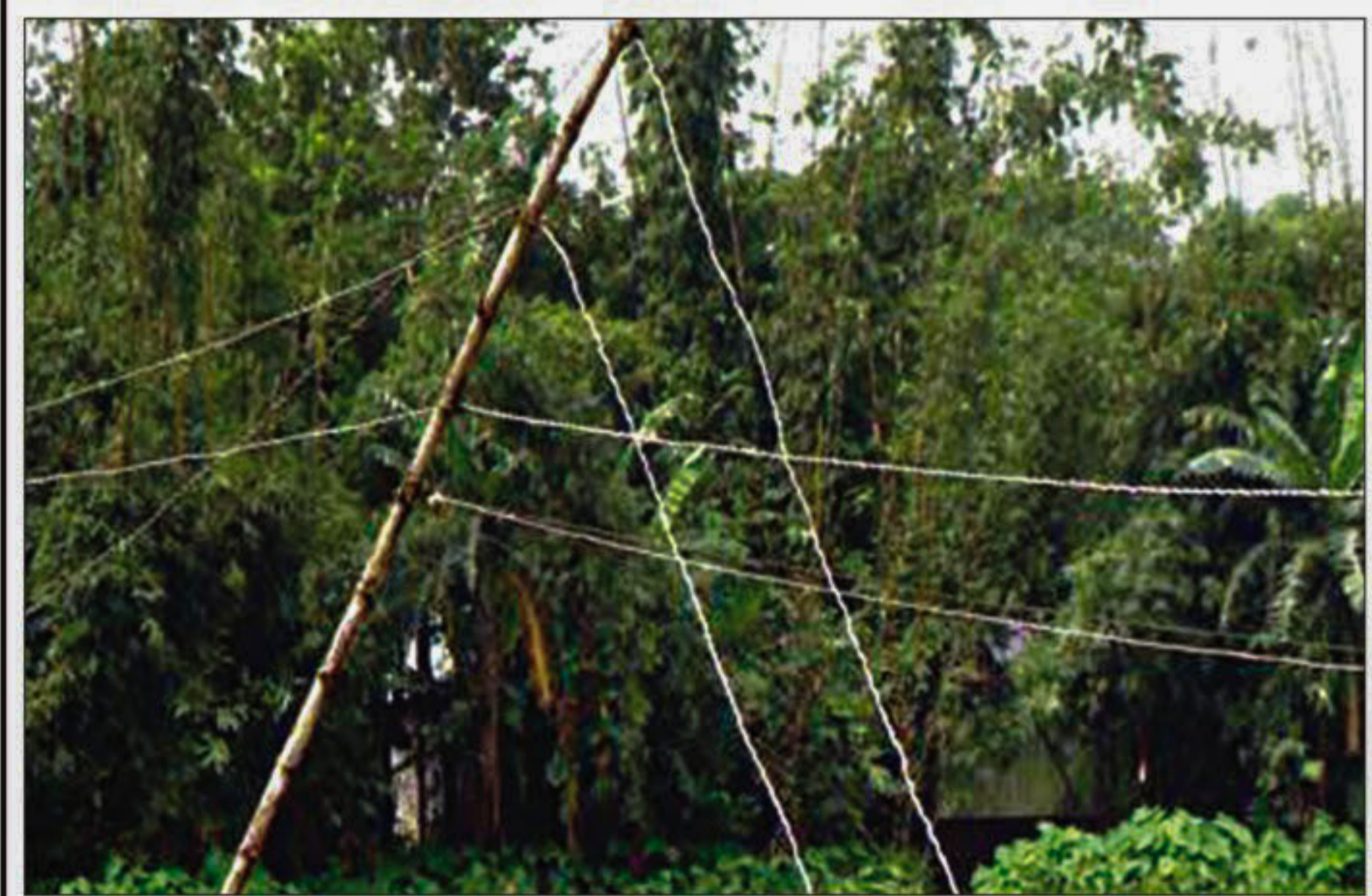
PHOTO: STAR Bare electric wires set in a dangerously slanting bamboo pole at Kholahati in Gaibandha Sadar upazila pose serious risk of accidents as a section of local Power Development Board staff continue giving electricity connection for irrigation and domestic purposes without safety measures.
