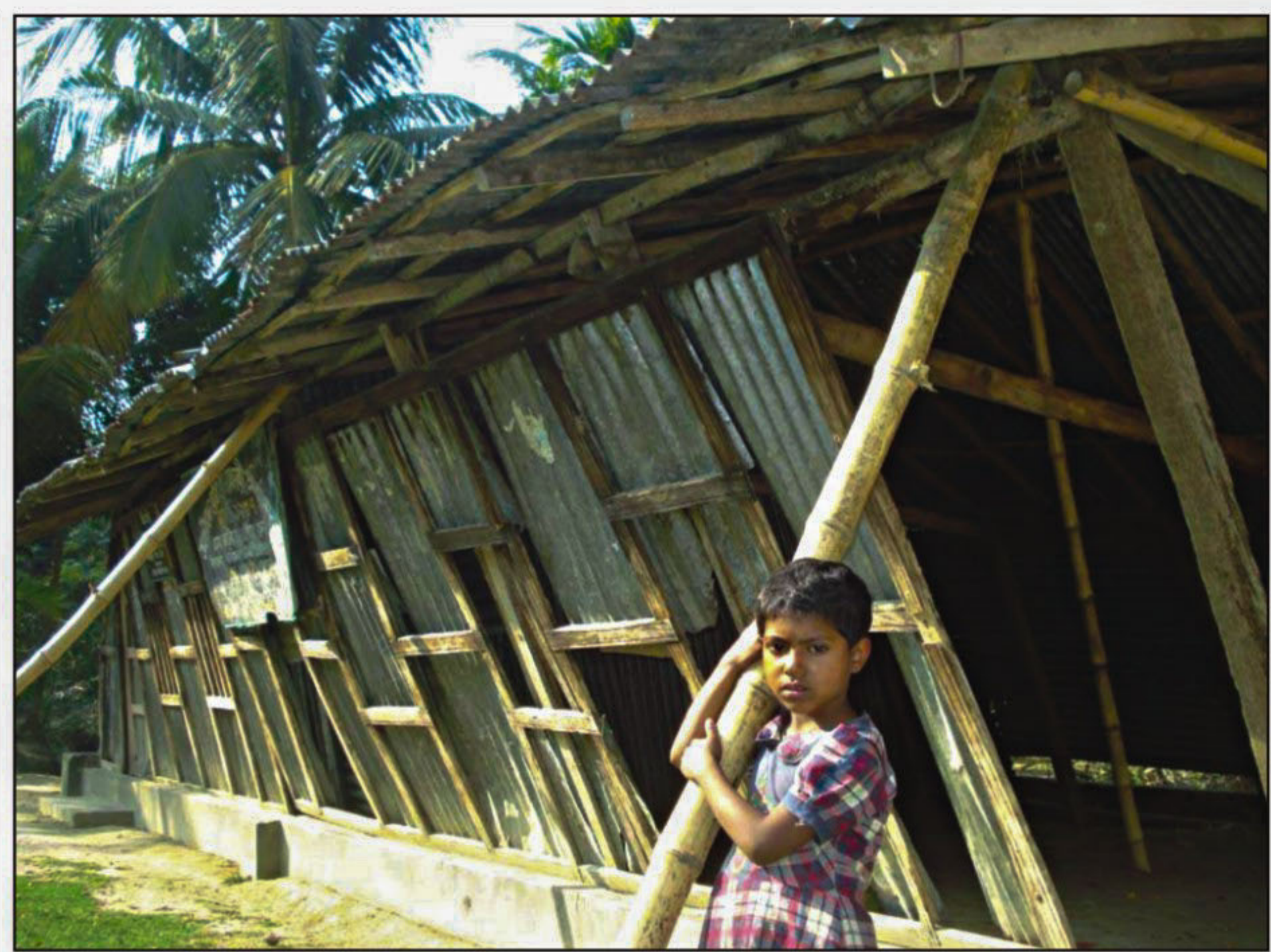
This non-government registered primary school at Batherhad village in Rupsa union of Faridganj upazila in Chandpur district remains in an awfully dilapidated condition, leaving over 200 students and four teachers vulnerable to accident anytime.
