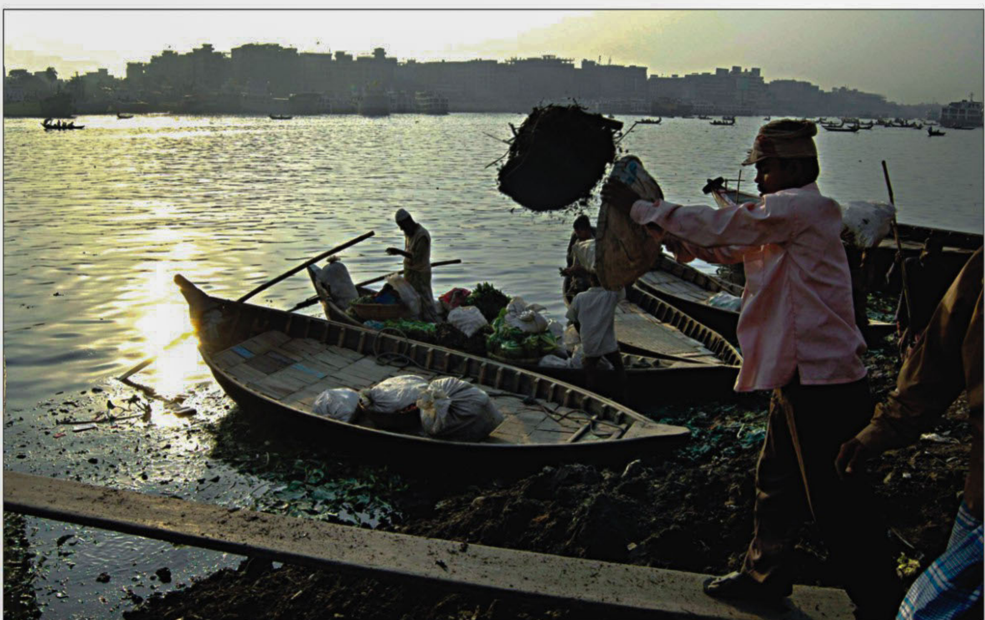
Workers constructing a jetty at Shyambazar of Farashganj in the capital yesterday dump soil into the Buriganga when authorities concerned are conducting a drive to clean up the river. Dumping of garbage in the river goes unabated despite campaigns to save the lifeline of Dhaka. PHOTO: SHAWKAT JAMIL
