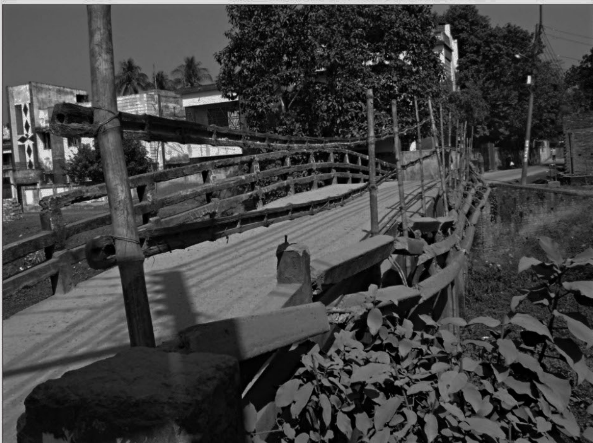
Awfully dilapidated Kadamtali Bridge across Ichhamati River at Kacharipara in Pabna town poses risk of accidents, especially at night, thanks to the indifference of authorities.
