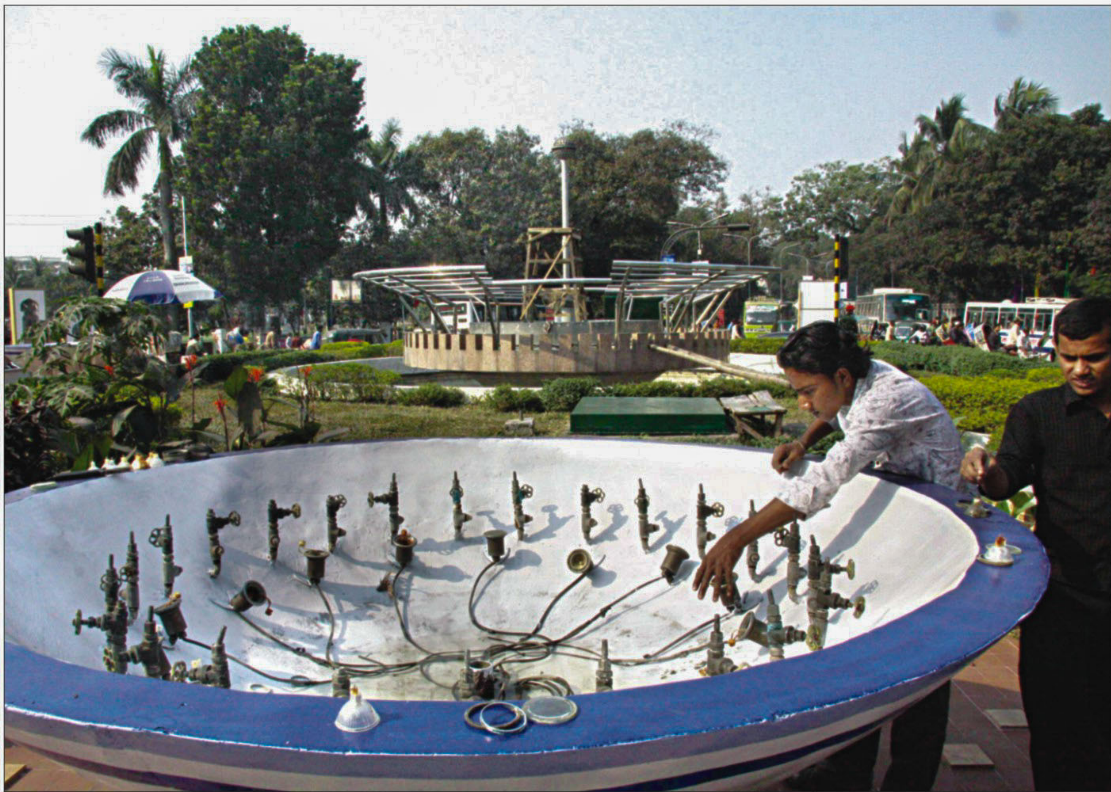
Refurbishment of Kadam Fountain in front of the foreign ministry in progress. Many such fountains are being renovated in the city ahead of SAF Games 2010 scheduled to begin on Friday. PHOTO: SK ENAMUL HAQ
