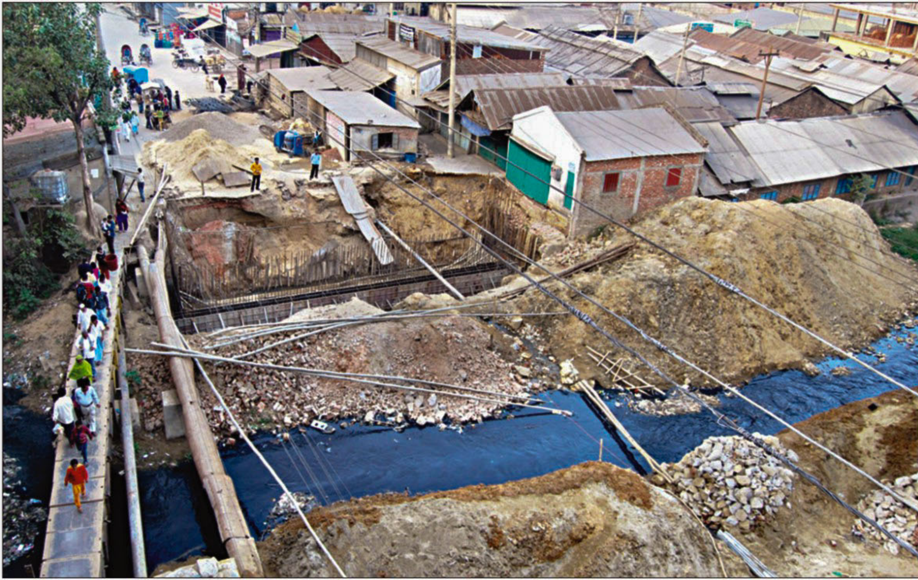
Pedestrians cross a makeshift bridge over Mirza canal on the Panchlaish-Muradpur road. Vehicular movement on the road remained suspended for the last eight months due to delay in construction of a bridge over the canal, causing immense suffering to the commuters.
