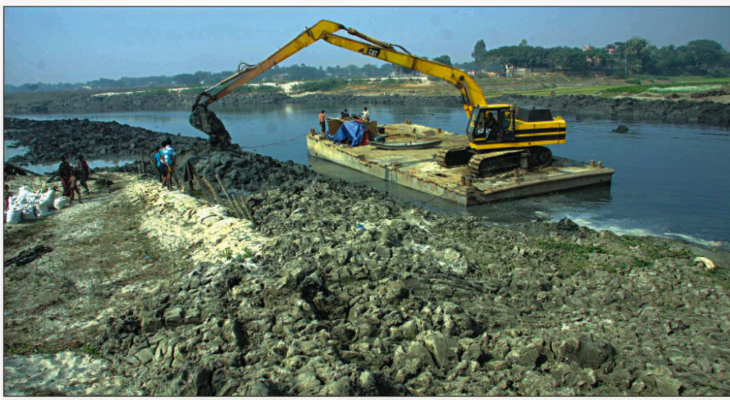
Bangladesh Inland Water Transport Authority excavates the Turag river as part of Dhaka Circular Waterways project. The photo taken recently shows a scavenger piling up soil removed from the riverbed right on the bank.
