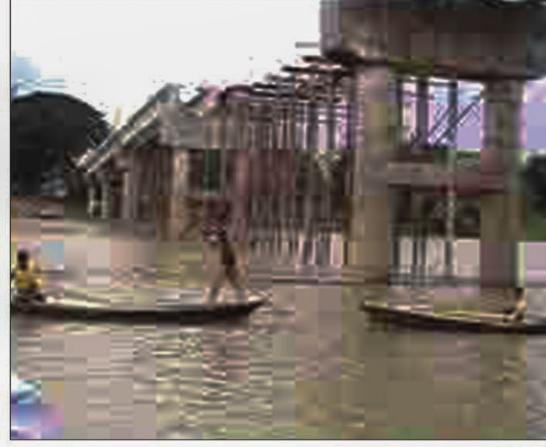
Fourteen years after start of construction, incomplete Shuknakuri bridge on Netrakona-Durgapur road in Durgapur upazila remains a farce for the local people who have to make tedious journey for going to other areas.
