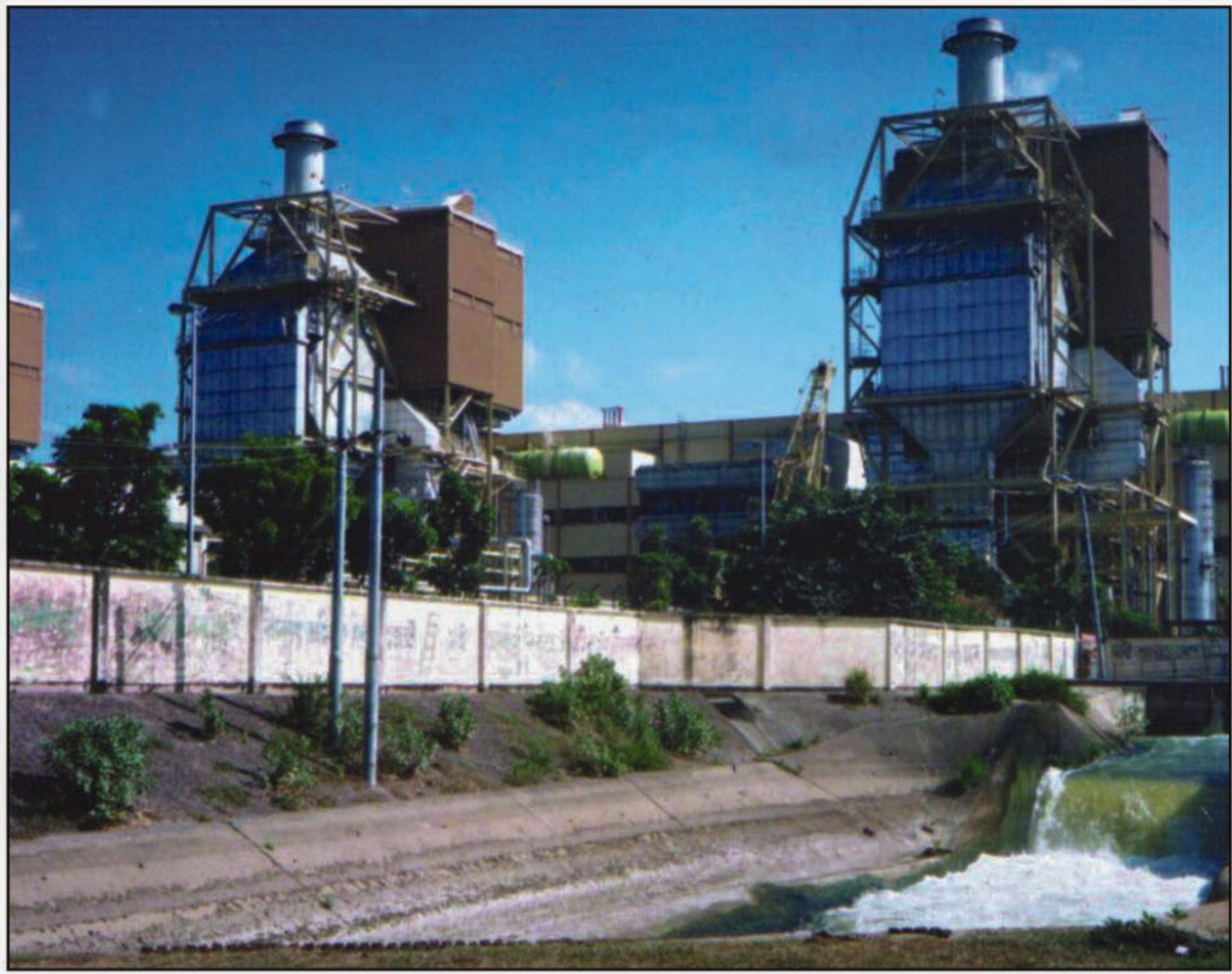
Ashuganj power station now limps with run-down machinery.
