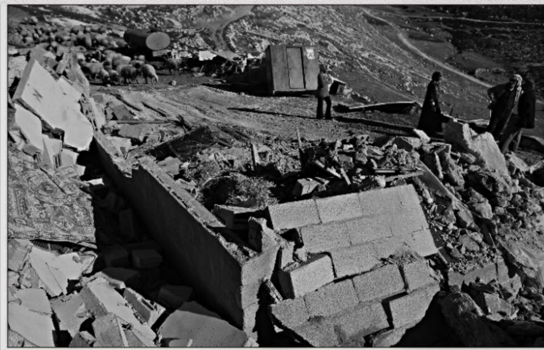
PHOTO: AFP Palestinians stand next to their demolished home yesterday in the farming village of Tana near Nablus in the so-called Area C, a closed military zone where Israel exercises full control.
