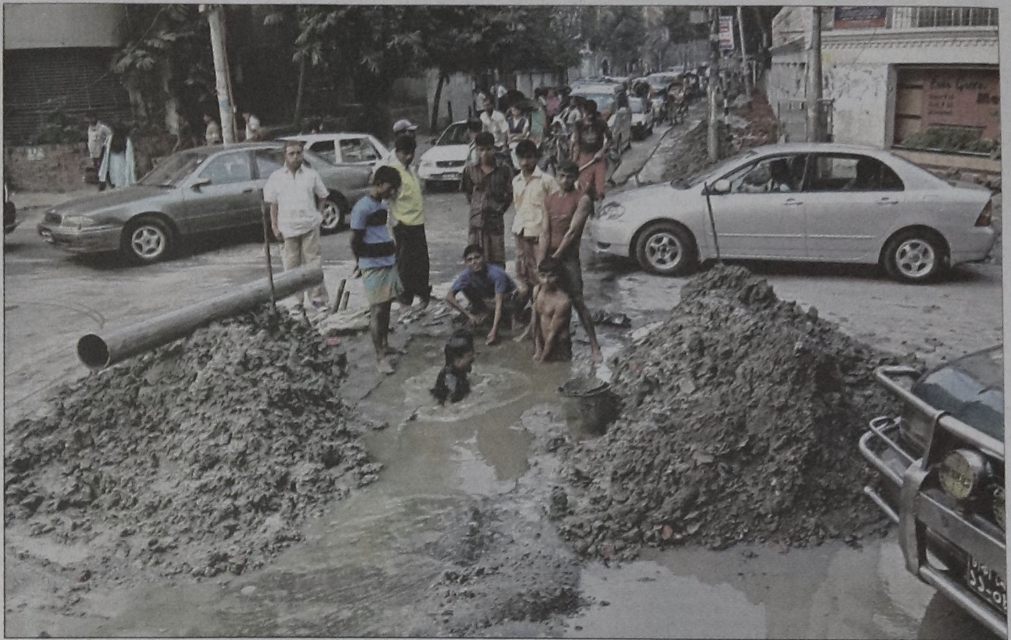
This photo taken at 7:40am yesterday on Dhanmondi 8/A road in the capital shows that vehicles carrying mostly school goers are facing trouble due to on going installation of Wasa pipelines. PHOTO: SHAWKAT JAMIL
