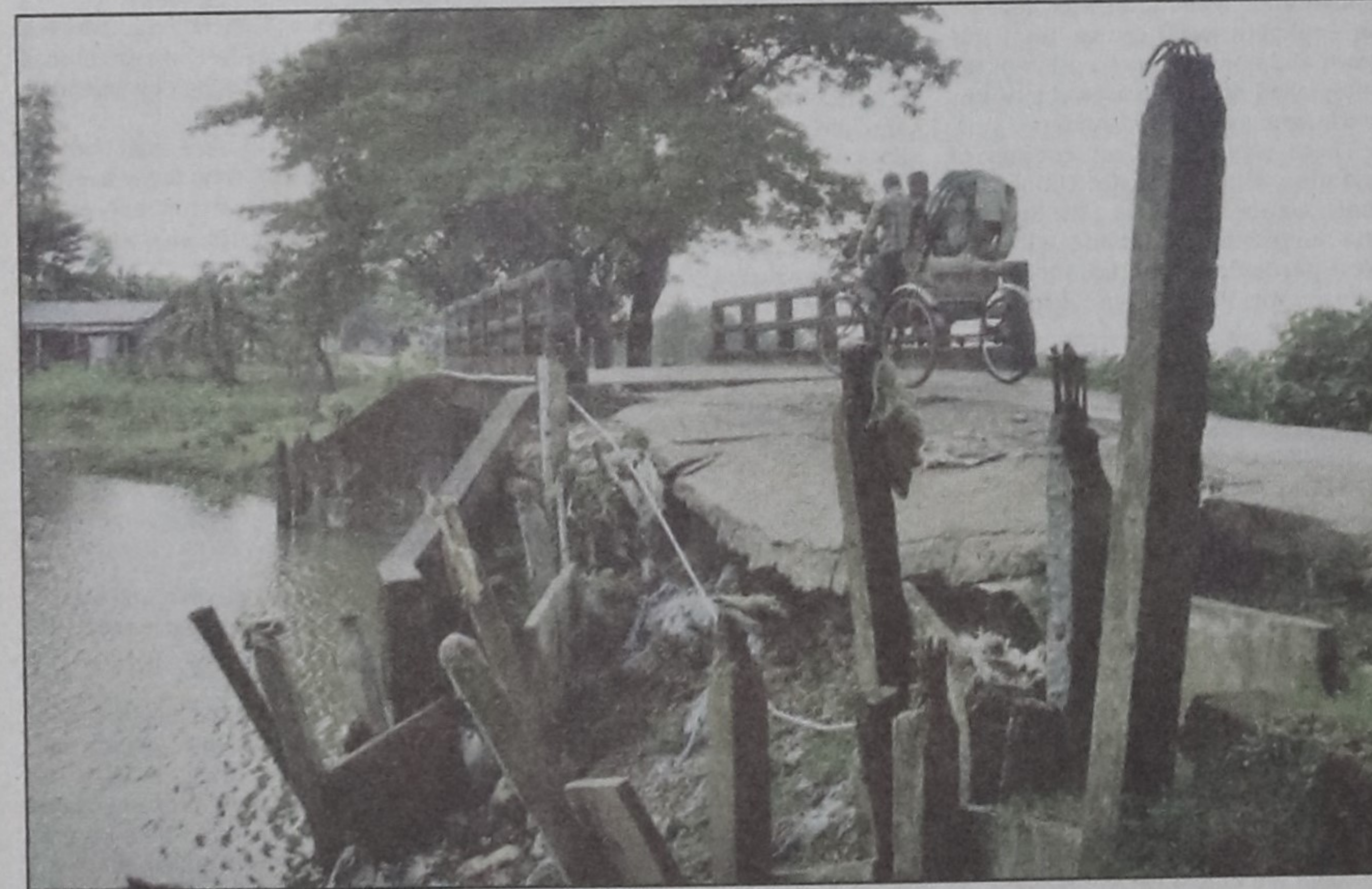
Threatened by erosion, this ramshackle bridge at Nabinagar in Sunamganj municipality poses risk for the commuters.
