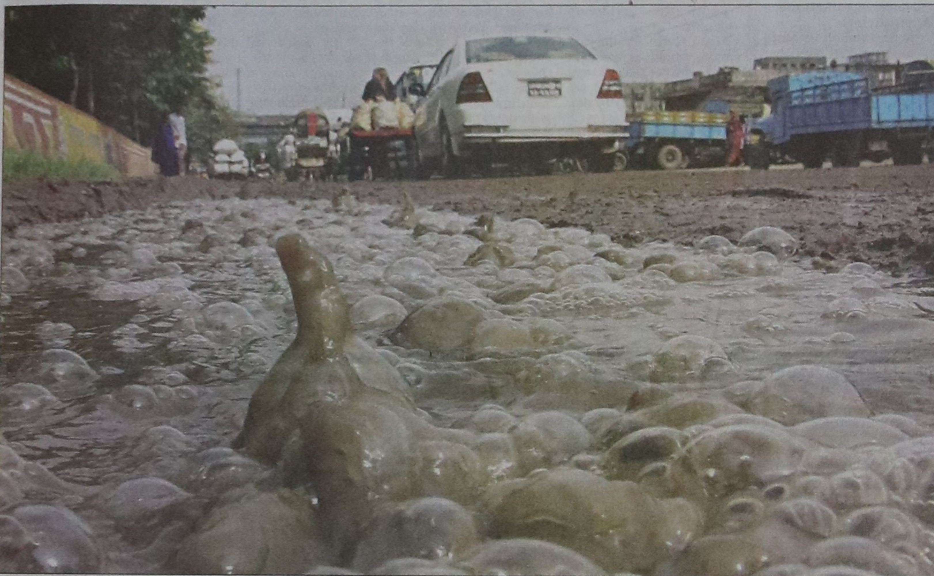
A leak in an underground gas pipe emits gas through a puddle on a road in Pagla in Dhaka yesterday. Locals claimed this has been continuing for almost the last two months.
