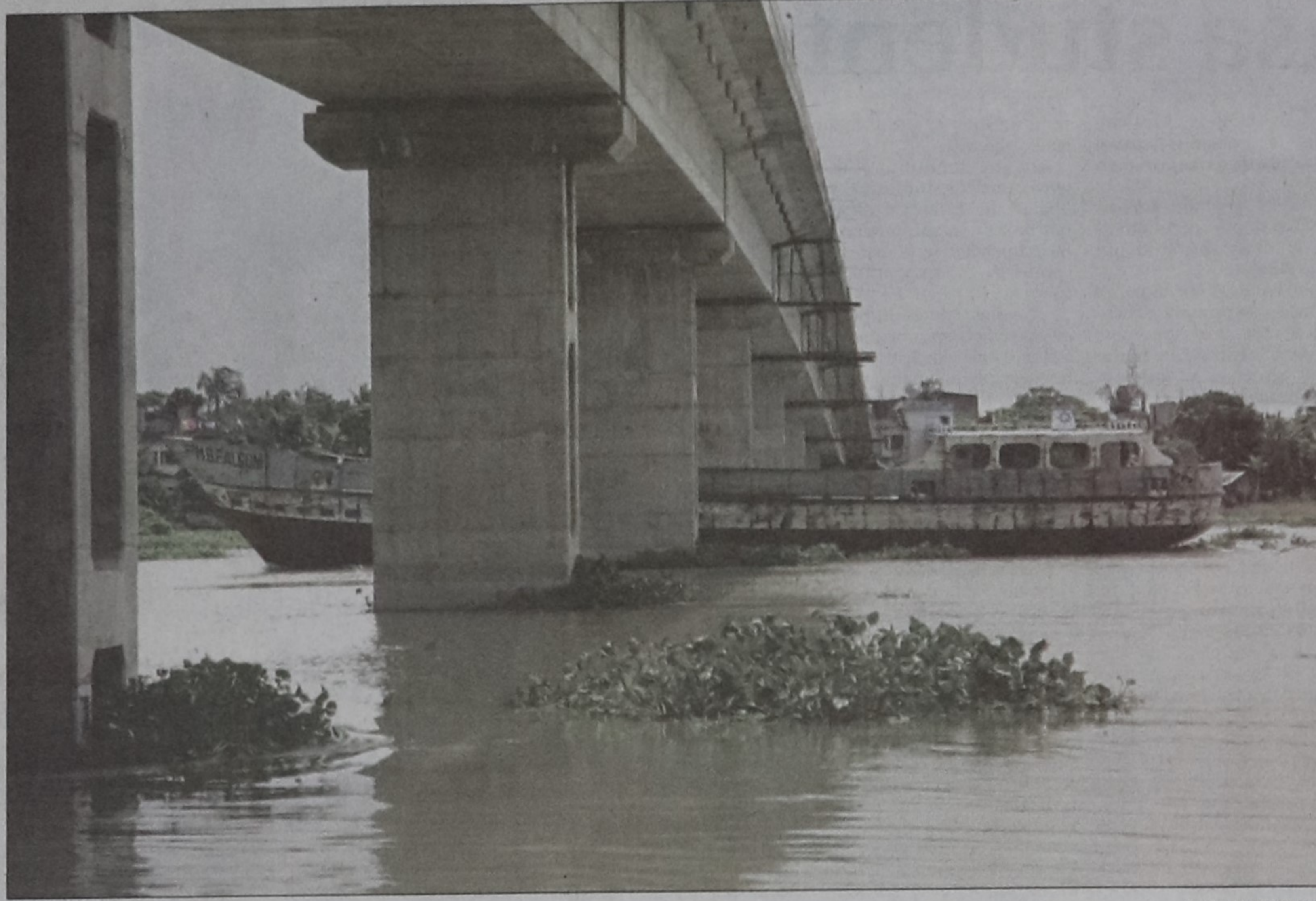
The cargo vessel got stuck while passing under the Third Buriganga Bridge as the bridge is being built two metres below the contract prerequisite.
