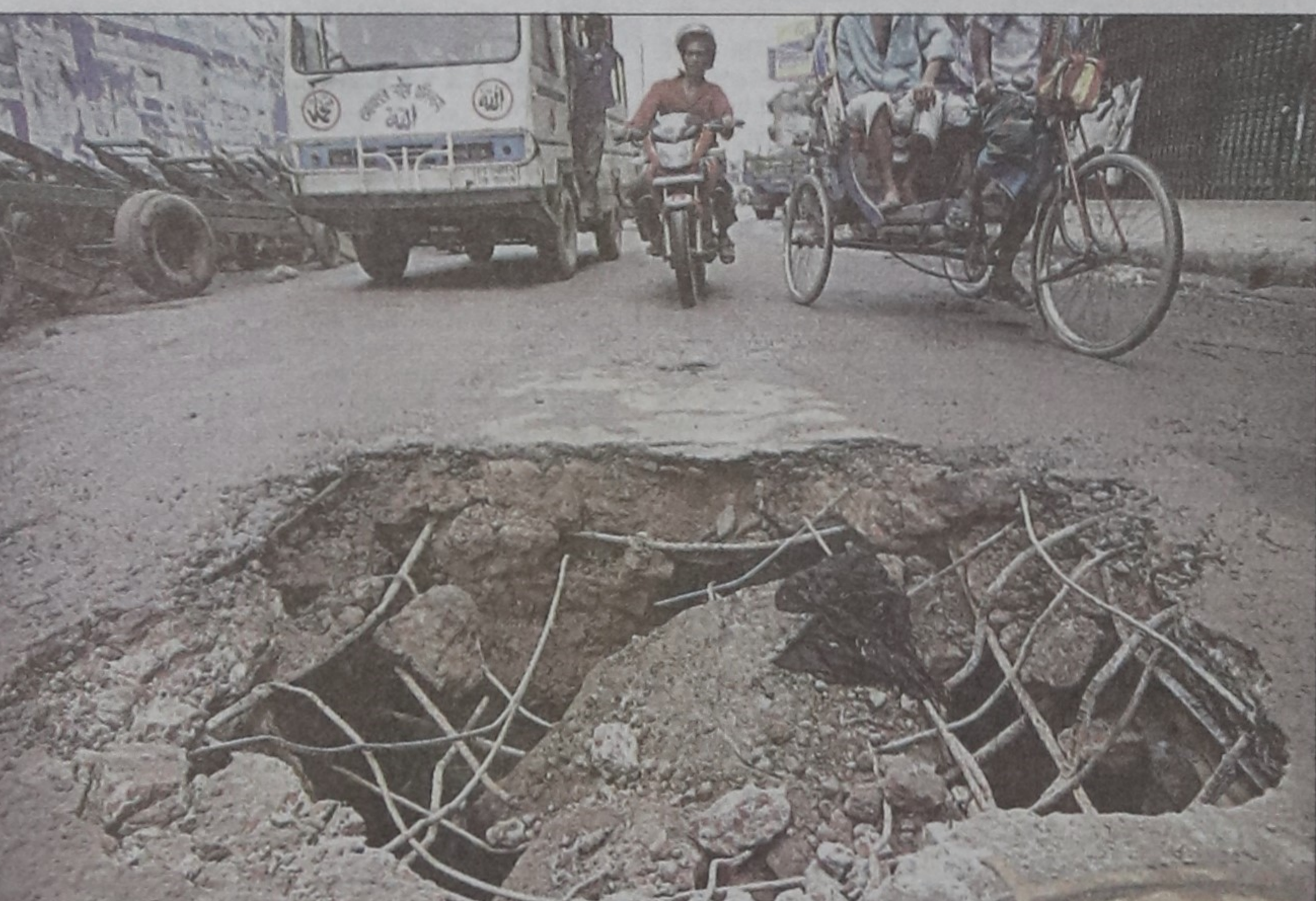
This motorbike rider sees the unmarked gaping hole on Babubazar Road in Old Dhaka at the last moment and manages to avoid an accident. The poor condition of city streets is reflected elsewhere in Dhaka as well.
