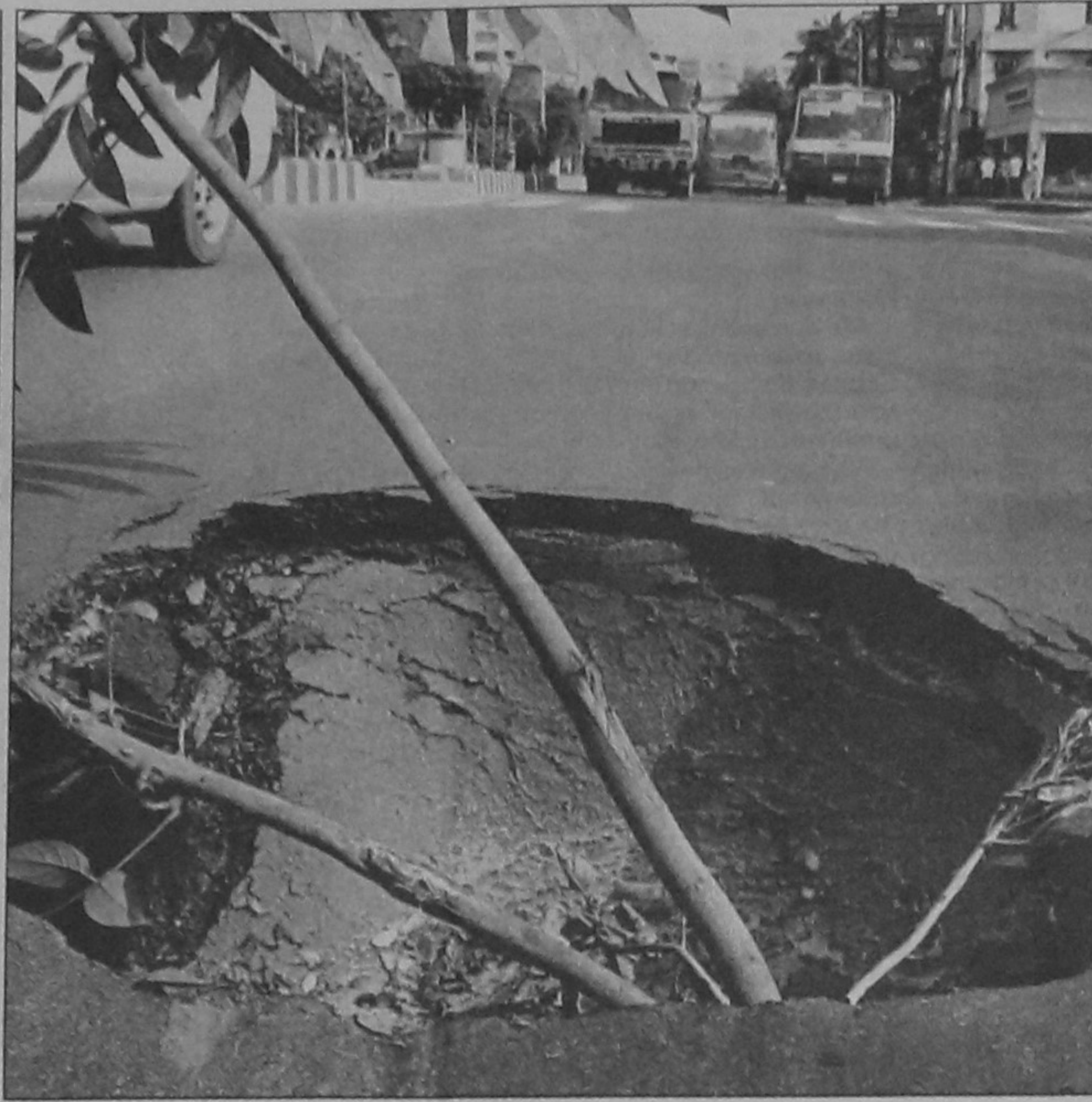
A massive pothole developed in the middle of the VIP road in front of Tejgaon Police Station on the airport in the city, making the movement of vehicles risky. The photo was taken yesterday.
