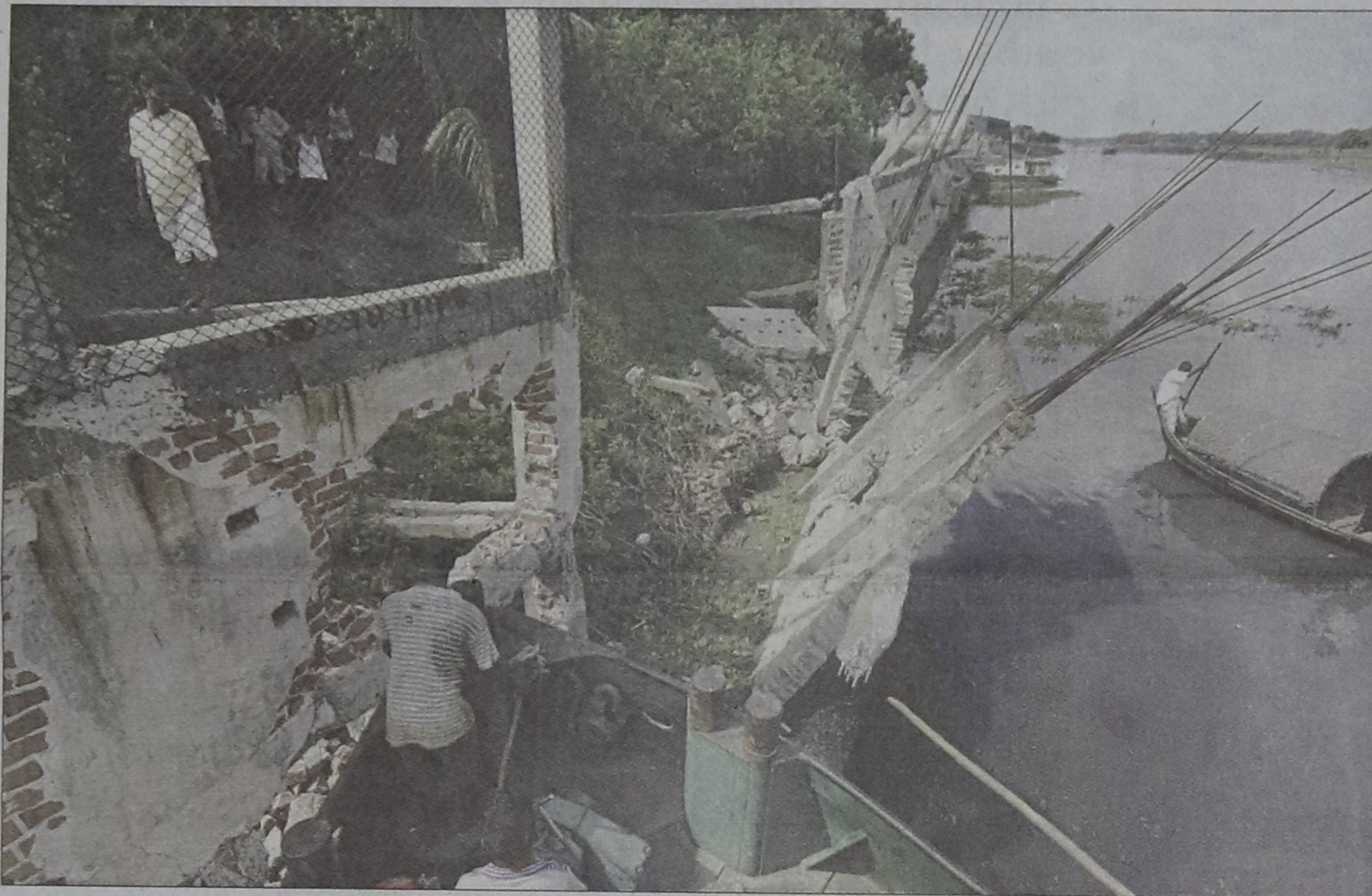
BIWTA workers yesterday continue their demolition of the wall of The Merchant Ltd, which was erected encroaching on the Turag at Pagar of Tongi.
