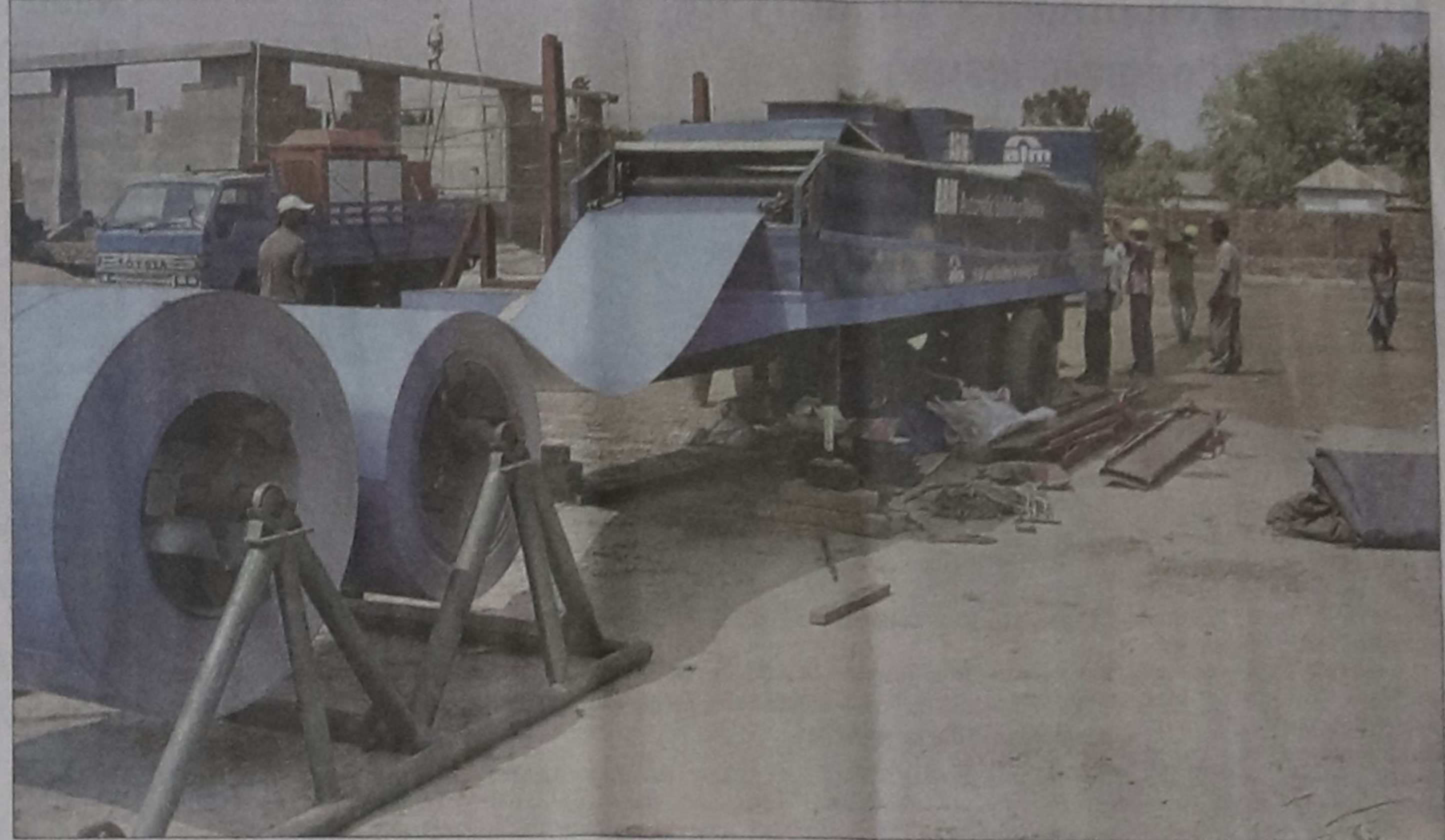
Steel coil is being shaped in line with the customer requirements at a construction site. ALM Steel Building Technology Ltd has brought in Automatic Building Machine technology to construct an infrastructure within a short span with a small manpower and lower costs.
